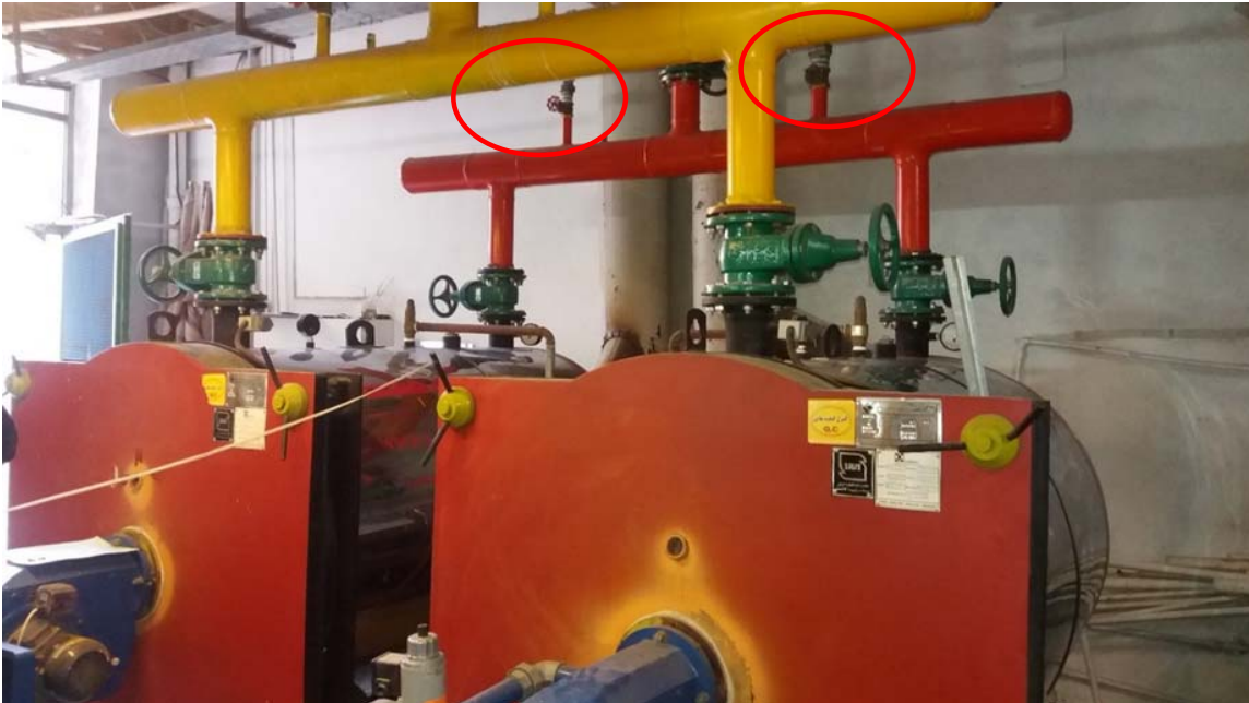
Fig. 6: Valve in the direction of the pipe connection of the expansion vessel to the boilers
