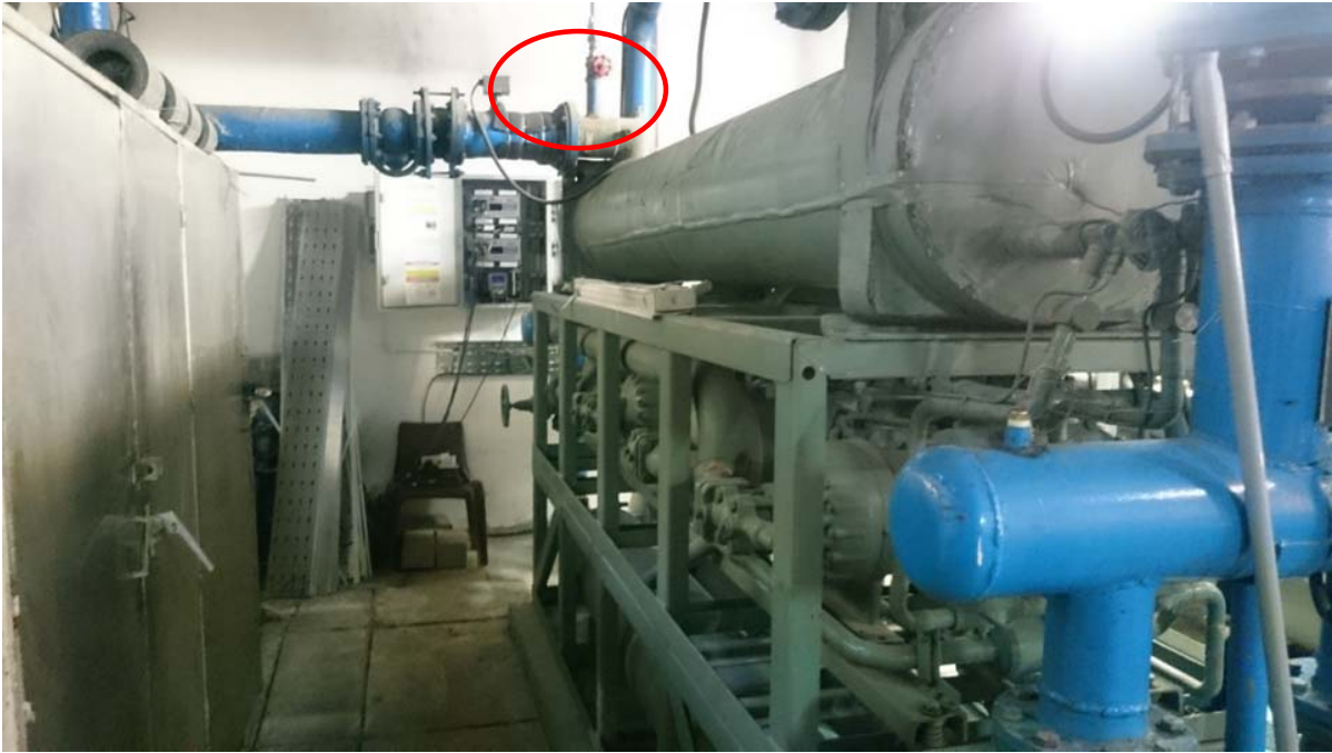
Fig. 5: The presence of valve in the pipe connection pipe expansion line to chiller No.1
