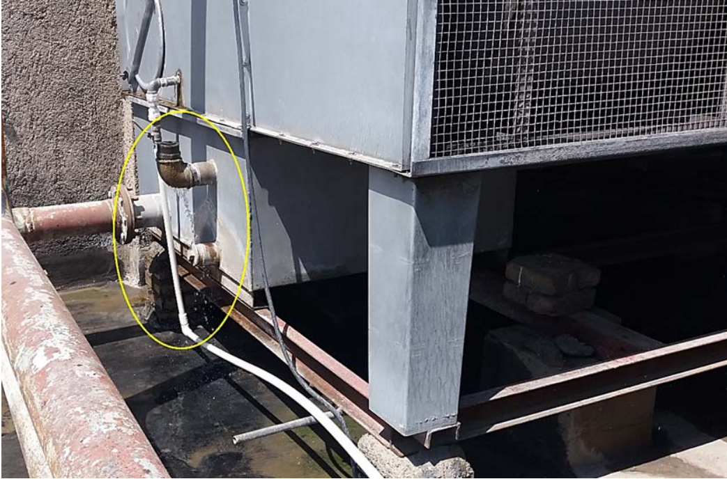
Figure 1. Water overflow from the cooling tower
