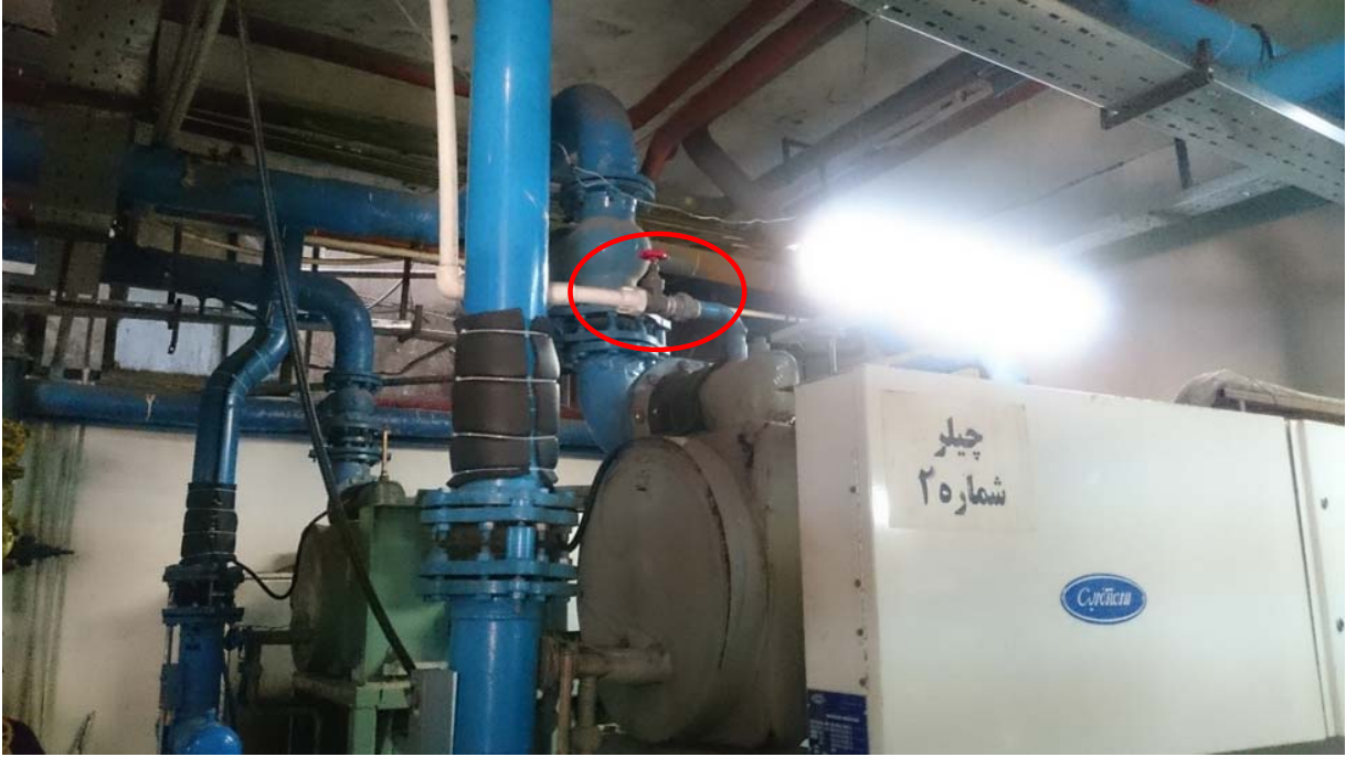
Fig. 4: Valve in the pipe connection pipe to the expansion chiller No. 2
