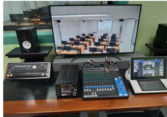
e-Learning classroom control panel
