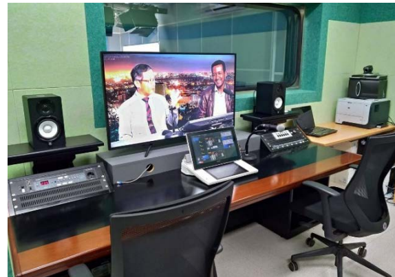
Studio control equipment
