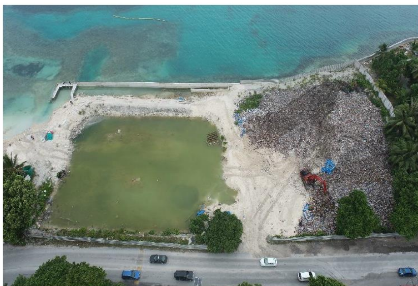
Figure 2: showing Cell 1 at the right, being filled, and Cell 2 at the left, under construction
