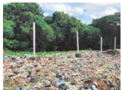
Vertically extended landfill gas venting pipes
