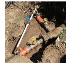
Bypass line & Flow meter
