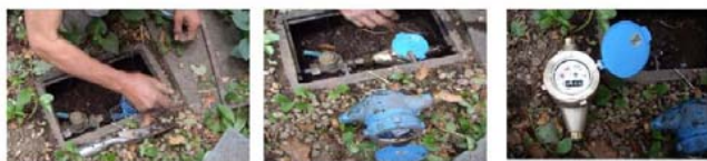
Replacement of old water meter in 8th year New meter (13mm R-100)
