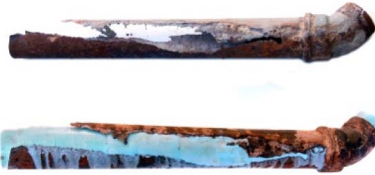
Electrolytic Corrosion of mild steel pipe
