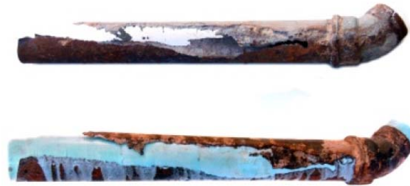
Electrolytic Corrosion of mild steel pipe
