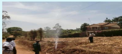
Leakage from bad connection point
