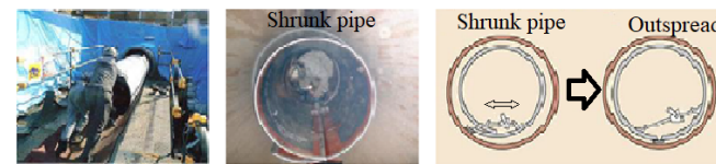
Figure-21 Image example of the method of inserting new Shrunk pipe (800 mm or more)
