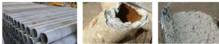
Figuer-37 Damaged Asbestos-cement Pipe
