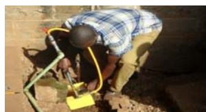
Handpump use for new connections 17
