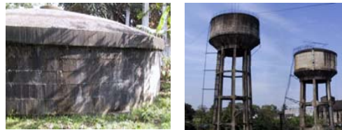
Figure-3 Example of a concrete-type distribution reservoirs
