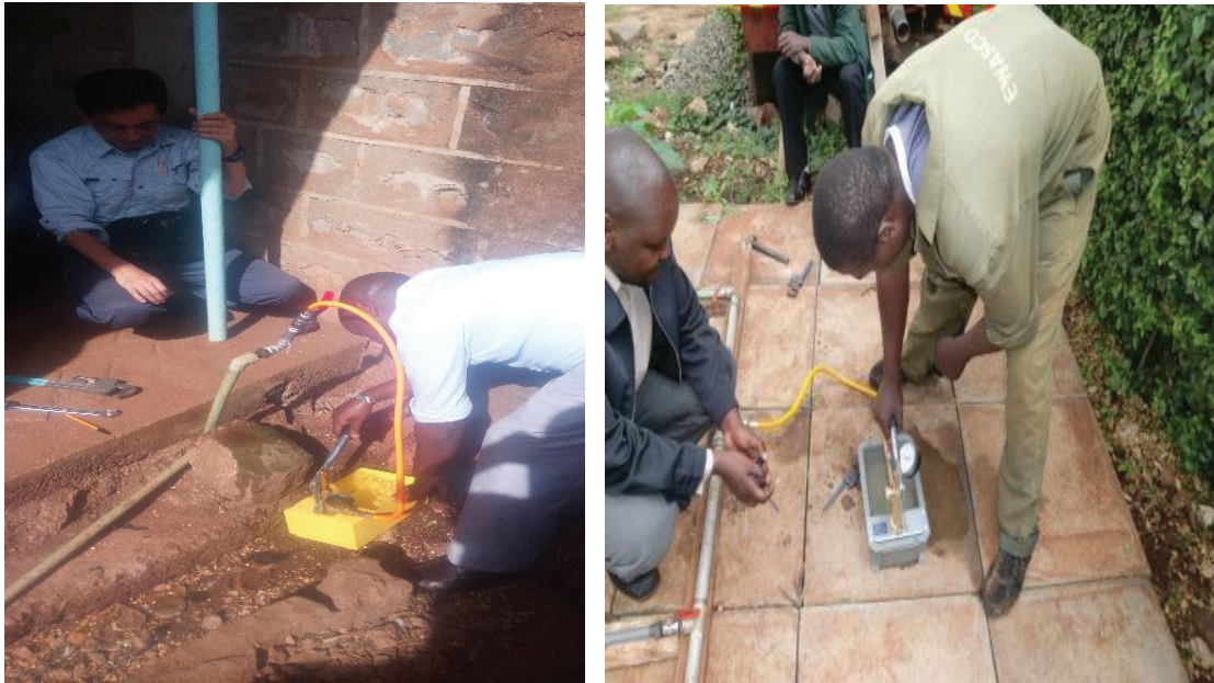
Figure 7.1: Hand pump connected on different pipe materials ready for use
