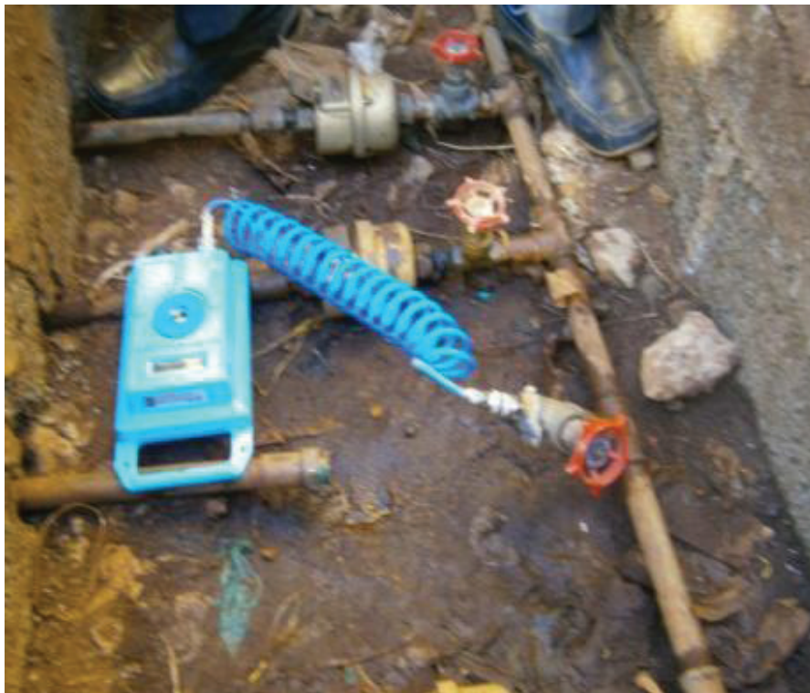
Figure 6.6: Pressure Logger Installed on Pipe
