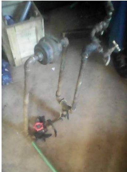
Illegally bypassed meter discovered by KEWASCO
