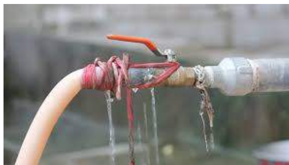
Leakages at connections are very common
