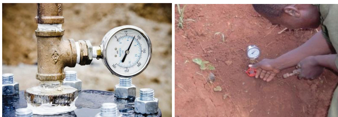
Figure 6.2: Pressure gauges installed on pipes
