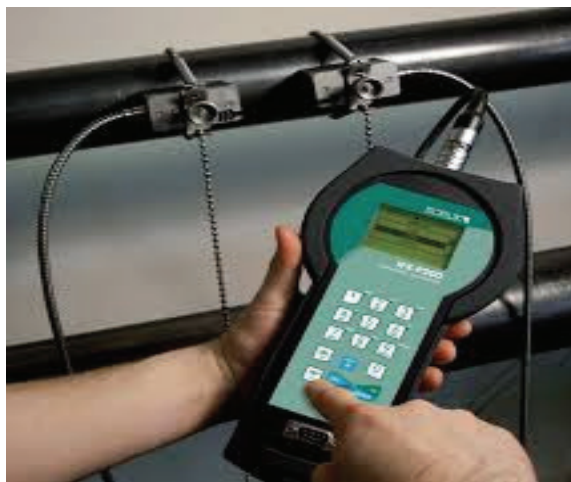
Figure 5.15: Side-mounted sensors on PVC pipe
