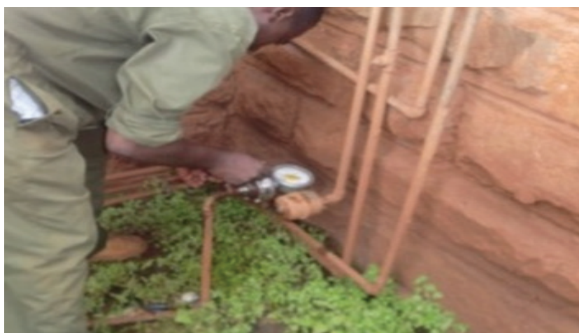
Figure 6.3: Pressure gauge installed at customer metering point
