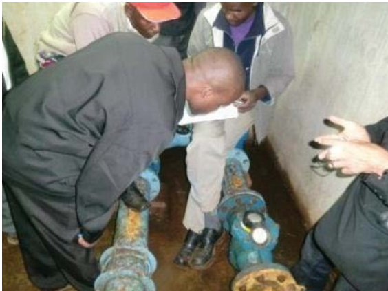
Figure 9.8: Flow Meter Reading
