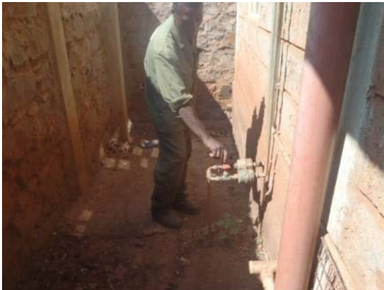
Figure 8.5: Close all peripheral valves of the block and all the customer valves completely
