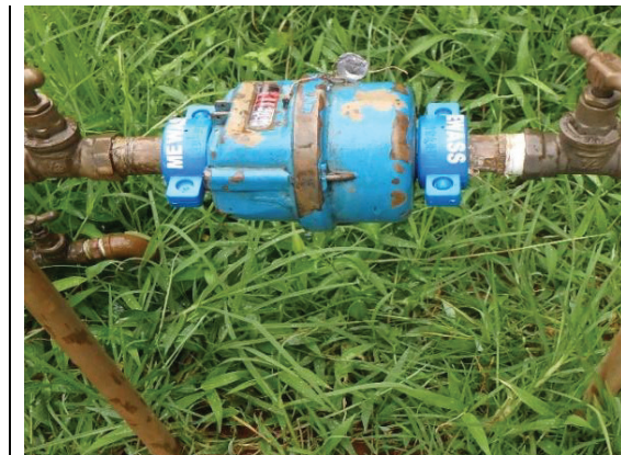
Figure 8.12: Meter Sealed Using Plastic Seals
