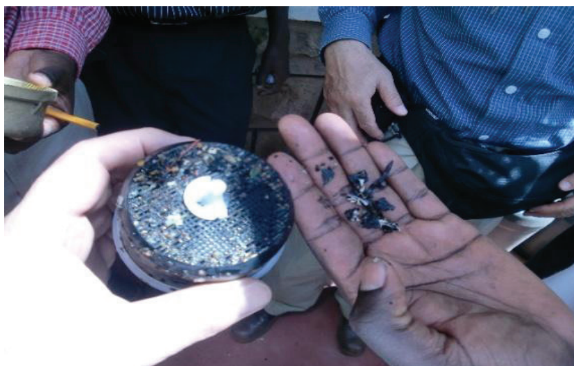
Figure 8.3: Debris trapped meter strainer
