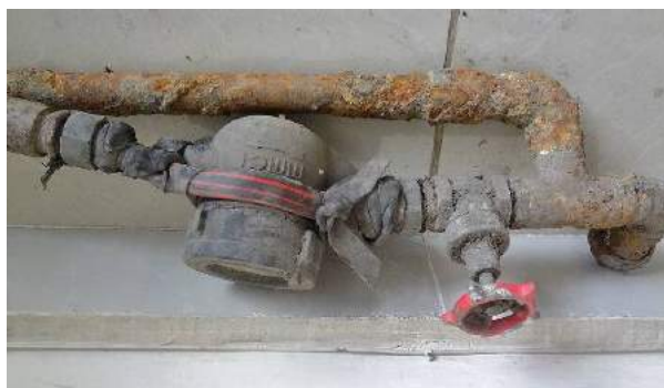
Example of water theft with modified pipe to bypass the meter
