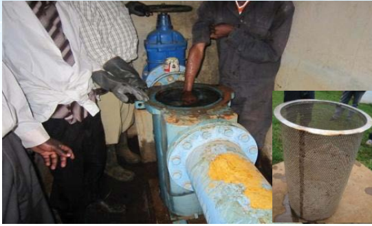
Figure 6.1: Strainer (Installed at outlet of Water Treatment Plant) (Meru WSP)
