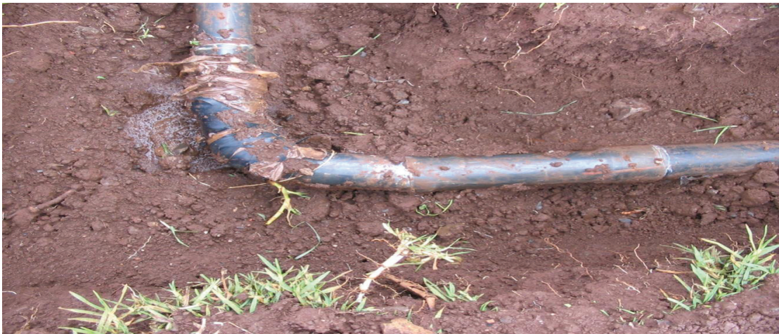
Figure 2.15: Poor Repairs with Fire-made Couplings
