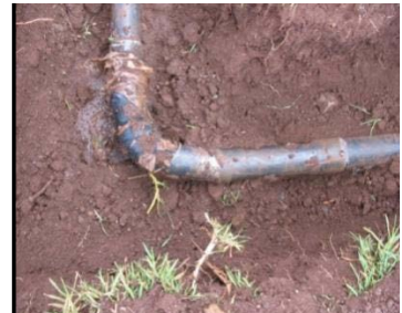
Figure 8.10: Plastic Pipe Bend (used for pipe connections in Kenya)
