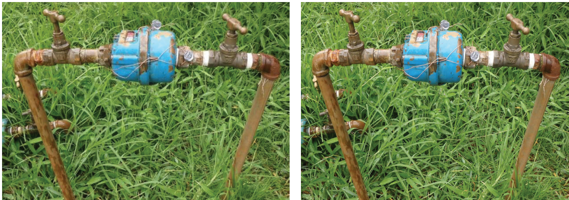
Figure 8.8: Meter sealed by sealing wire and sealing lead
