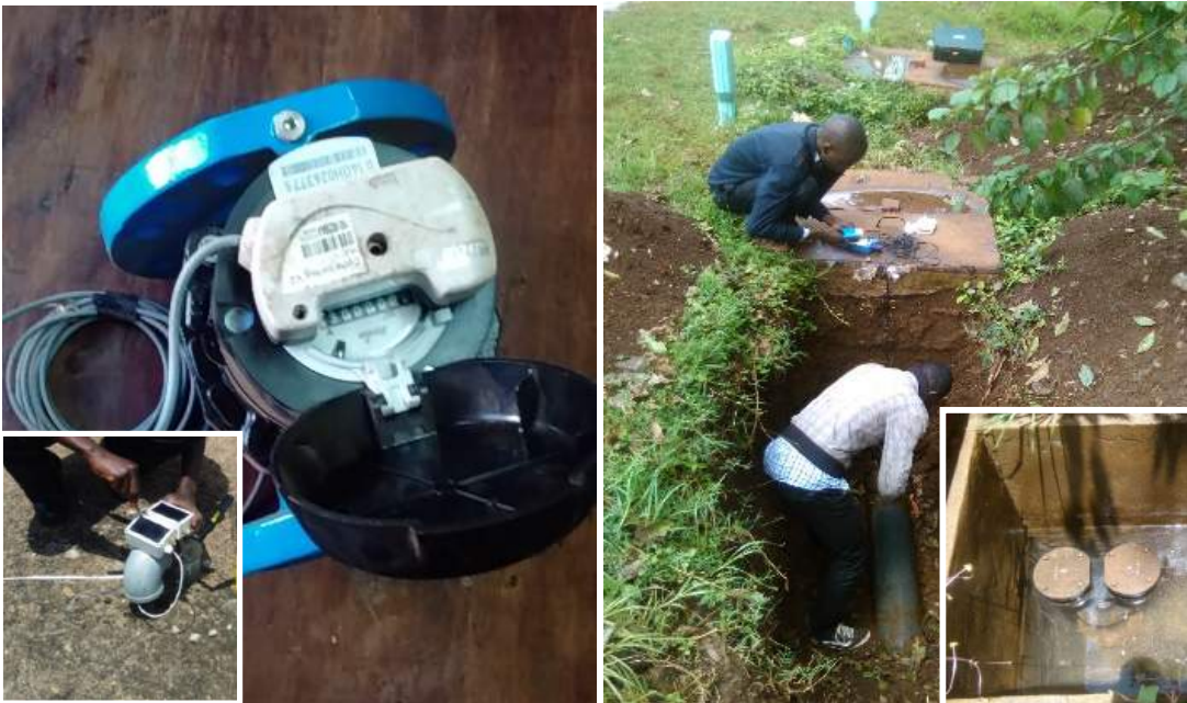
Left - typical flow sensor and data logger installation at KEWASCO, right- set up of ultrasonic flow measurement device
