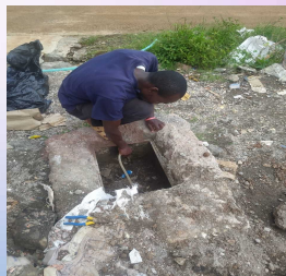
No meter at a connection
