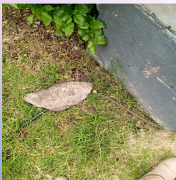
Connection By-passed meter
