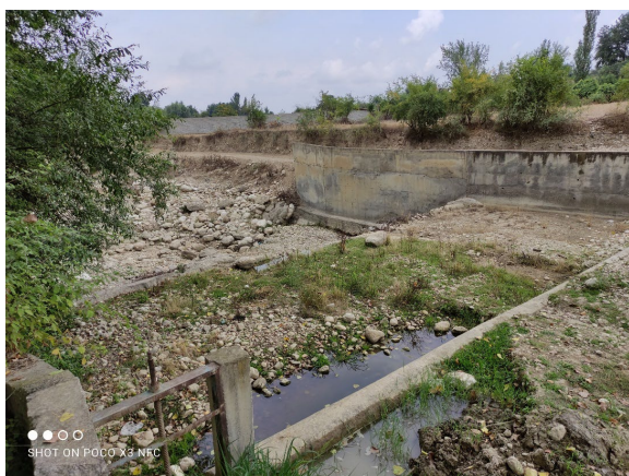
Fixed Weir on a Branch River (Gerankooch Area)
