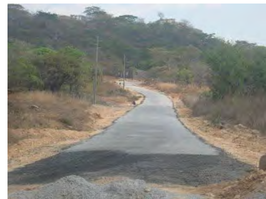
Poor quality of road compaction in progress
