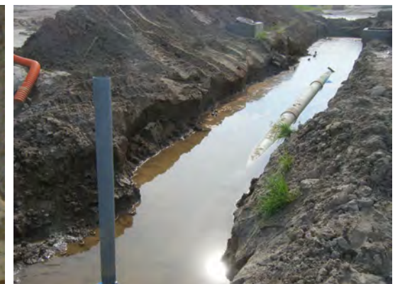
Watered pipeline lacking of protection
