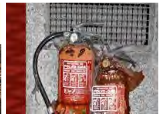
Corroded fire extinguishers
