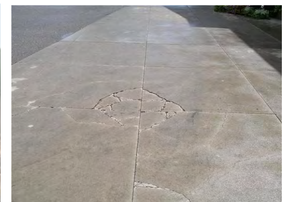
Results of poor compaction
