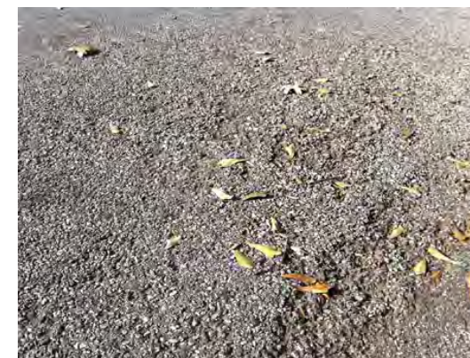
Raveling due to extremely porous asphalt
