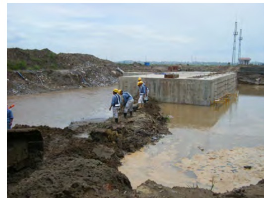
Water logging due to mis-sequence of construction plan
