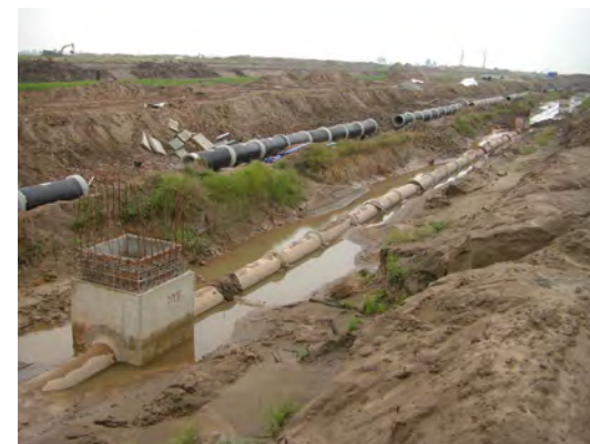
Mismanagement of buried pipe ①
