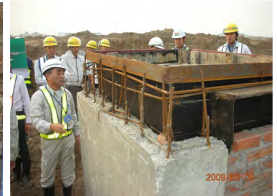
Failures due to unmanaged quality of building according to layout
