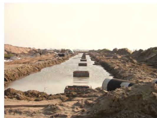
Water logging around the pillars under construction
