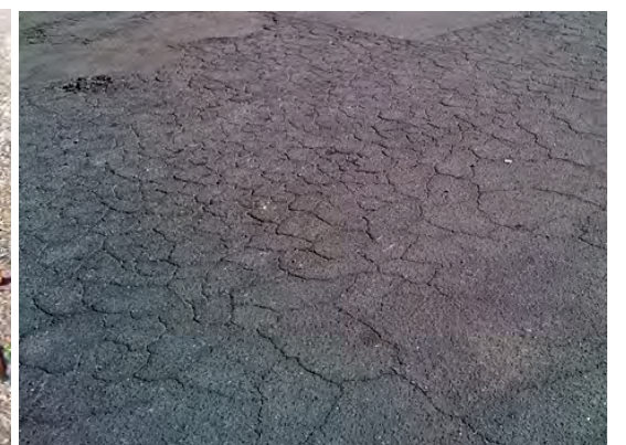
Alligator cracking due to low quality materials (asphalt)
