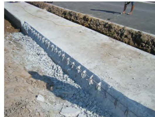
Uneven concrete works on pavement
