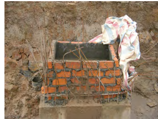
Defects in structure frame of pillar buildings
