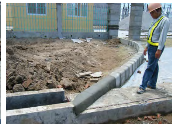
Misplacement of curbstone
