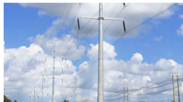
Figure 2-9 230kV Power Transmission Line
