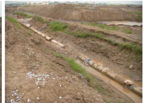
Mismanagement of buried pipe ②
