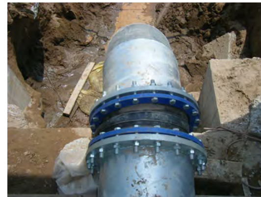
Poor bolting connection
