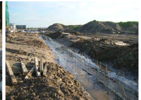
Mis-sequence of pipeline installation
