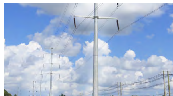
Figure 2-9 230kV Power Transmission Line
