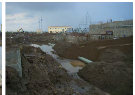
Water logging occurs during construction work for foundation
