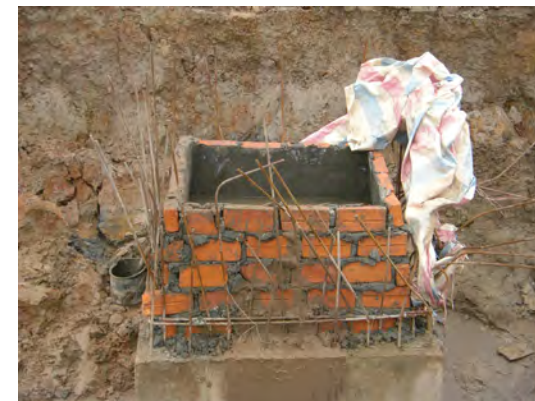
Defects in structure frame of pillar buildings
