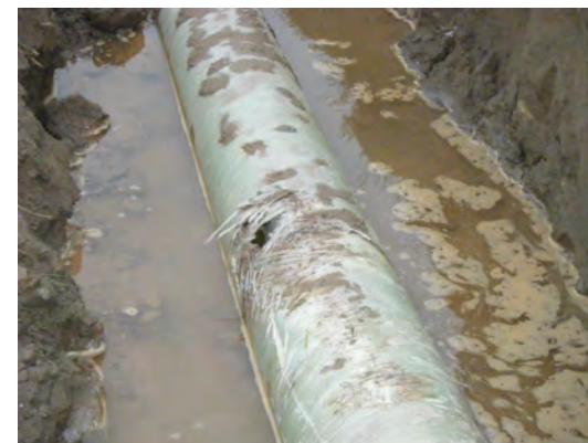
Hole that cause leaking in pipelines
