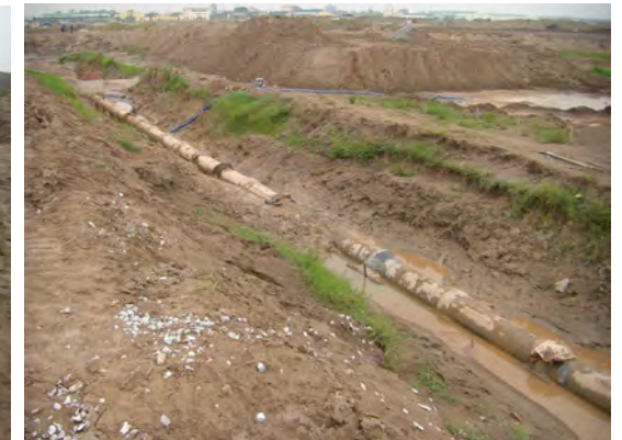
Mismanagement of buried pipe ②
