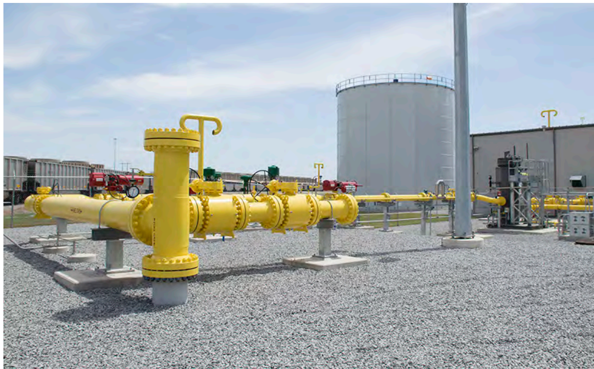
Figure 3-14 Gas storage tank and distribution pipelines
