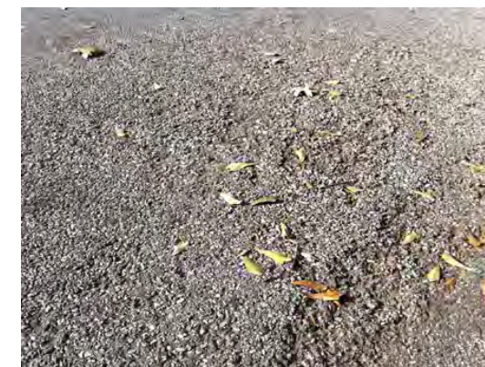
Raveling due to extremely porous asphalt
