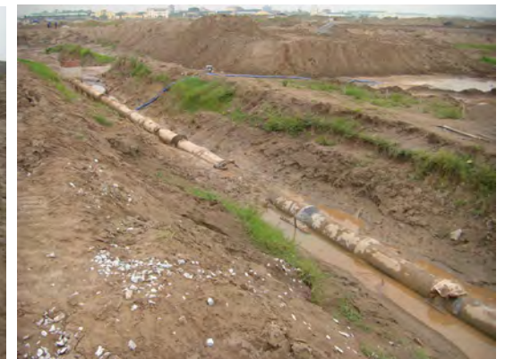
Mismanagement of buried pipe ②
