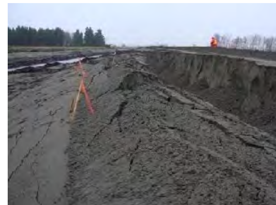
Failure of foundation on soft ground
