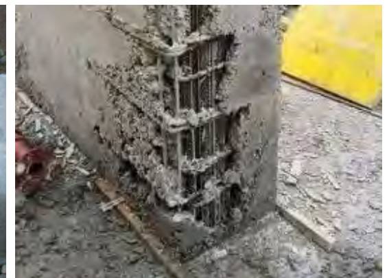
Honeycomb due to improper mix design
