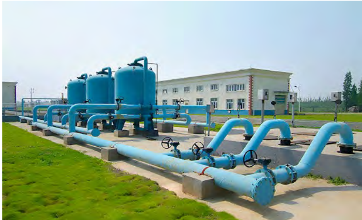
Figure 3-16 Water Treatment Facilities
