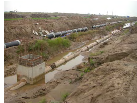
Mismanagement of buried pipe ①
