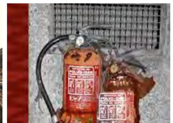
Corroded fire extinguishers
