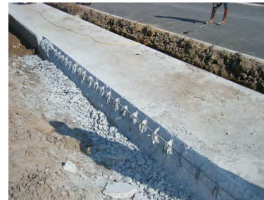
Uneven concrete works on pavement
