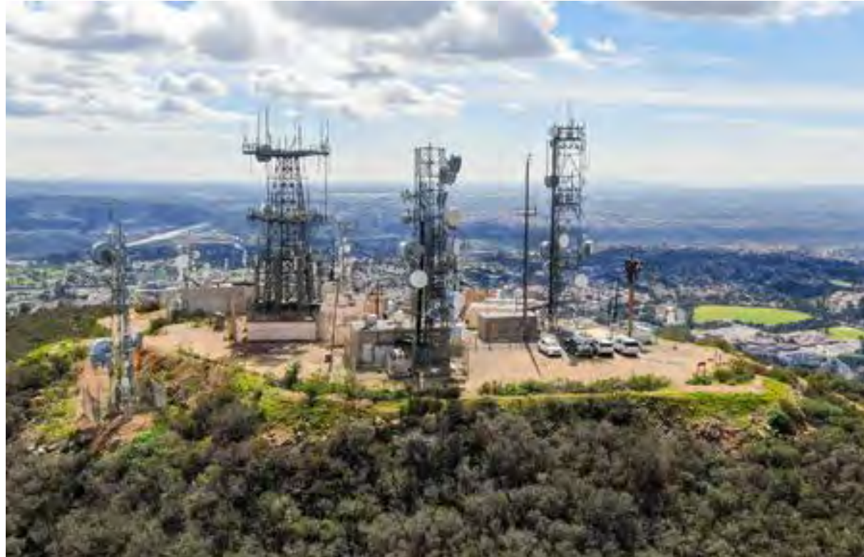
Figure 3-24 Transmitters of telecommunication facilities
