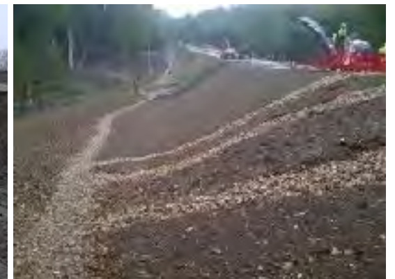
Failure during operation
