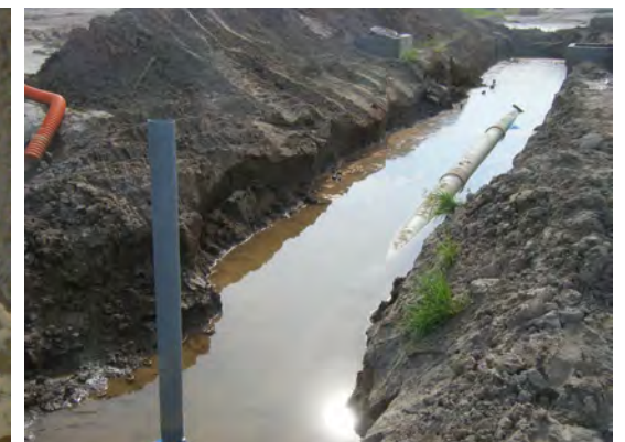
Watered pipeline lacking of protection
