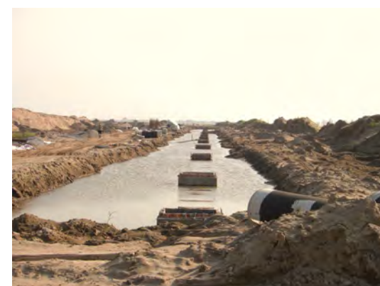
Water logging around the pillars under construction
