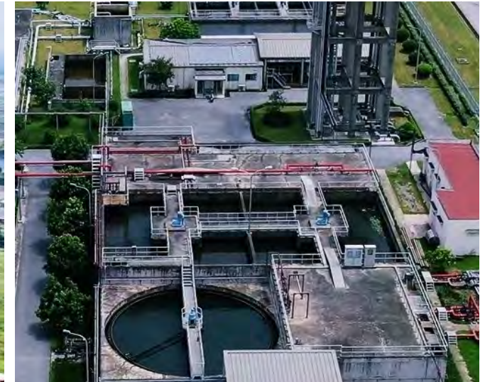
Figure 2-15 Water storage tank
