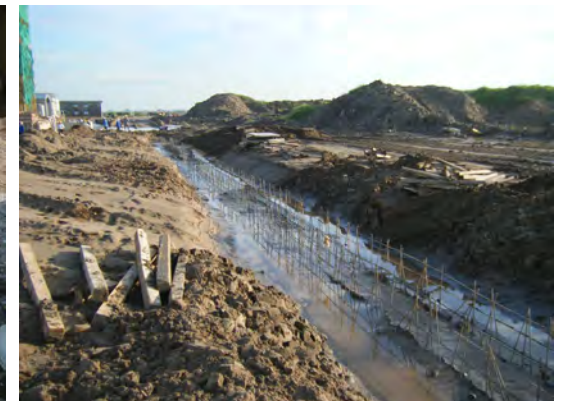
Mis-sequence of pipeline installation
