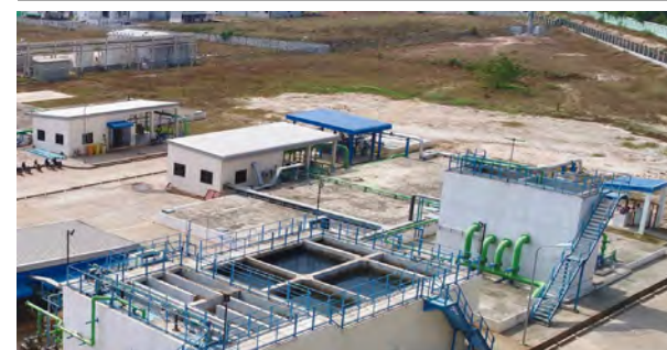
Figure 2-11 Water Purification Plant
