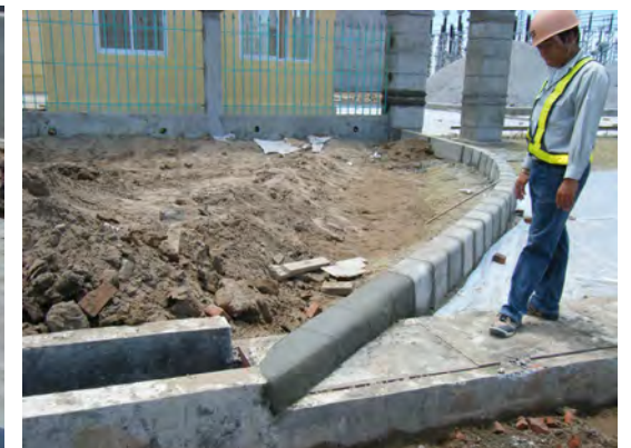
Misplacement of curbstone
