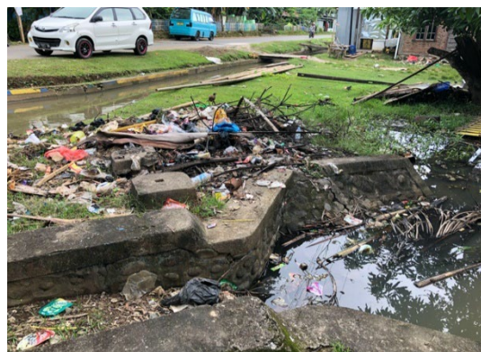
Example of domestic garbage dumped at the intake from a secondary canal to their tertiary canal
