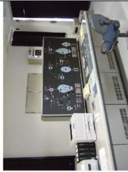
Supervisory Control And Data Acquisition system of the Underground Dam
