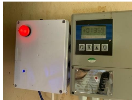
Electromagnetic Flowmeter Indicator (Rehabilitated Borehole)
