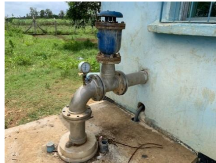
Pressure Gauge and Air Valve at Top of Borehole (New Borehole)
