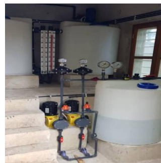
Disinfection Equipment in Mnarawambao Reservoir
