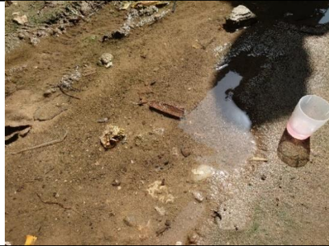
Photo 16: Detected water leakage The puddle was water leakage because residual chlorine was detected.
