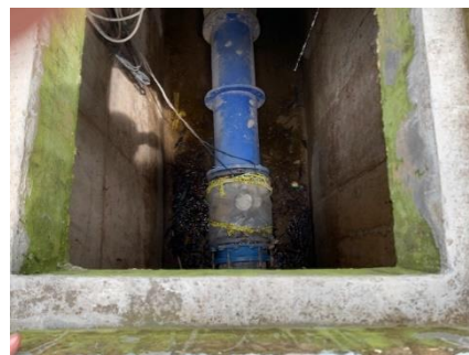
Flowmeter in Mnarawambao Reservoir
