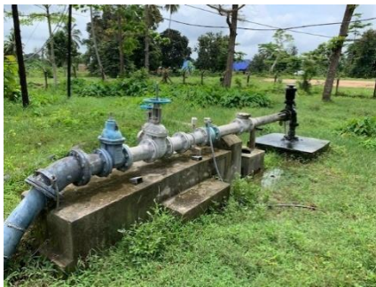
Piping Around Borehole and Leakage from Air Valve (Rehabilitated Borehole)
