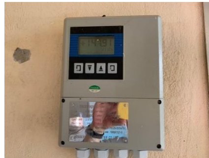
Electromagnetic Flowmeter Indicator (New Borehole)
