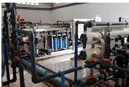
Photo 2.4 Reverse osmosis membrane (RO) filters
