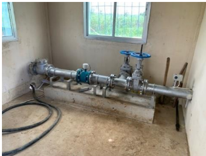
Piping and Flowmeter in Pump Room (New Borehole)
