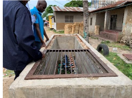
Manifold with Meters Already Installed
