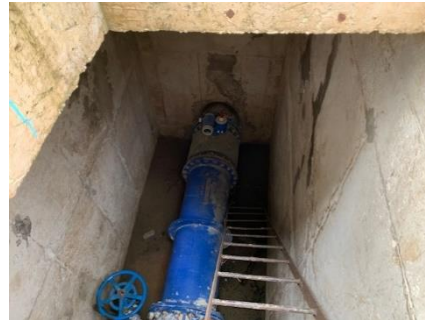
Distribution Flowmeter in Saateni Reservoir
