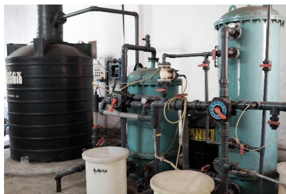
Photo 2.7 Reverse osmosis membrane (RO) filters
