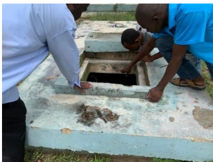
Flowmeter chamber in Mnarawambao Reservoir
