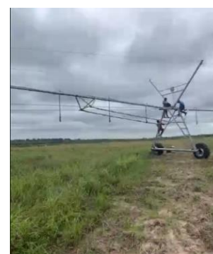
Photograph 6-15 Irrigation system (sprinkler) installed by a private seed production company
