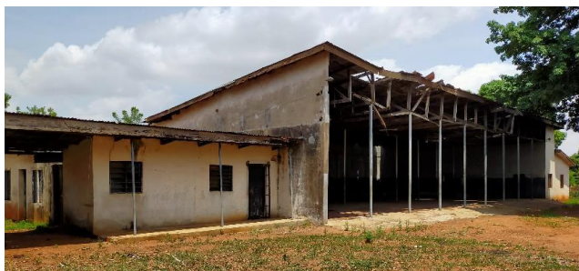
Photograph 4-19 Old machinery shed at the Nasarawa State Agricultural Office in Lafia
