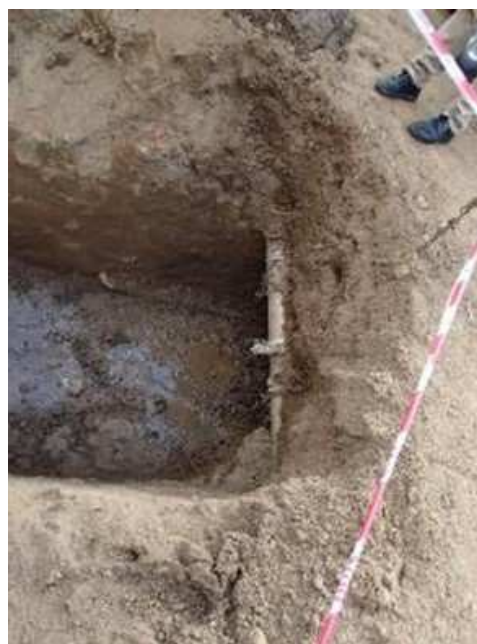
Figure 2-6.13 Deteriorated AC pipes
