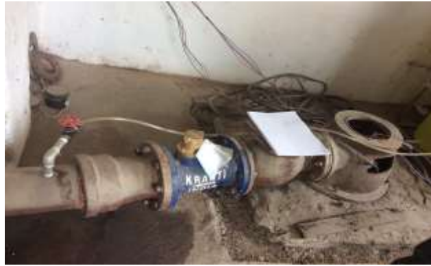
Flowmeter installed at samara WUSC Project-1
