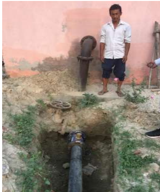
Flowmeter installed at samara WUSC Project-2
