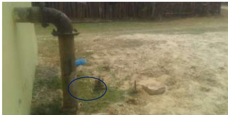
Flowmeter installed at deep tube well. Project-3. Valve chamber is under construction.
