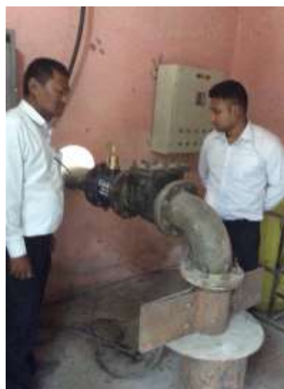
Flowmeter installed at samara WUSC Project-2
