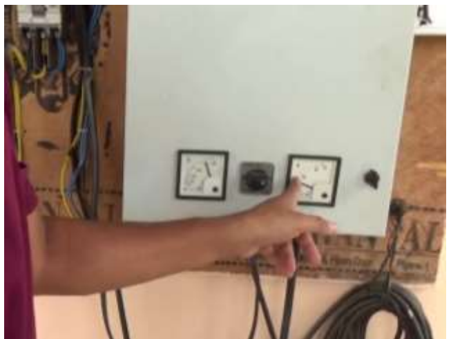
Photo-4. Checking Ampere/Voltage Meter
