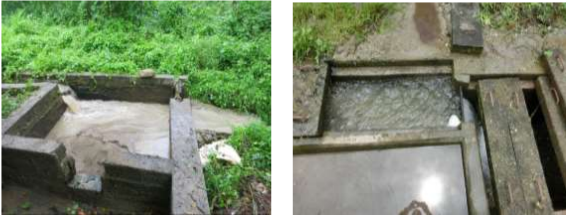
Figure 1.2 Typical Intake Structure (Left: Pragatinagar WUSC, Right: Dhulabari WUSC)
