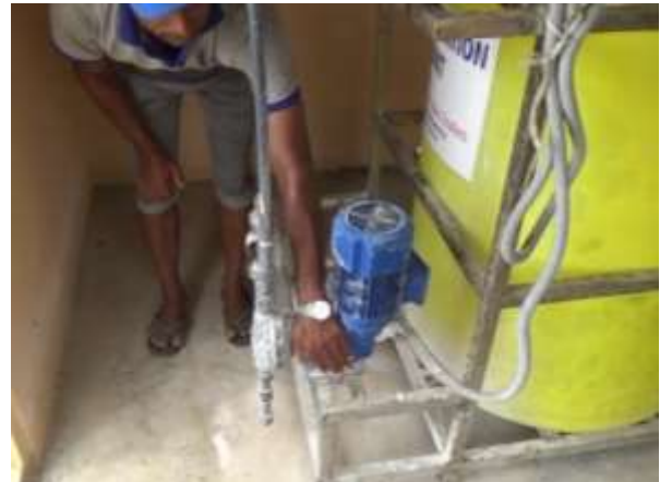
Photo 2.25 Daily Inspection of Pump (Abnormal noise and vibration)
