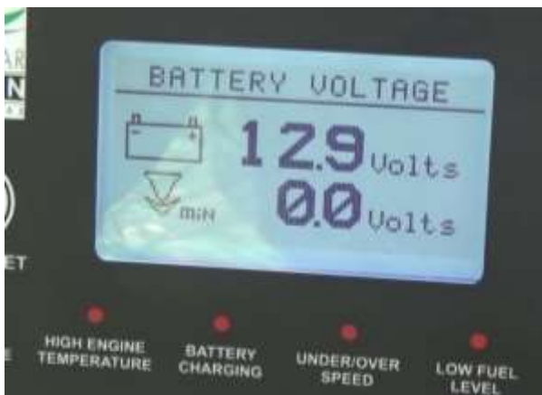
Photo 2.46 Checking Battery Condition
