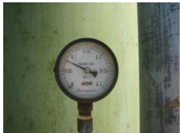
Photo 2.55 Pressure Gauge of Tank
