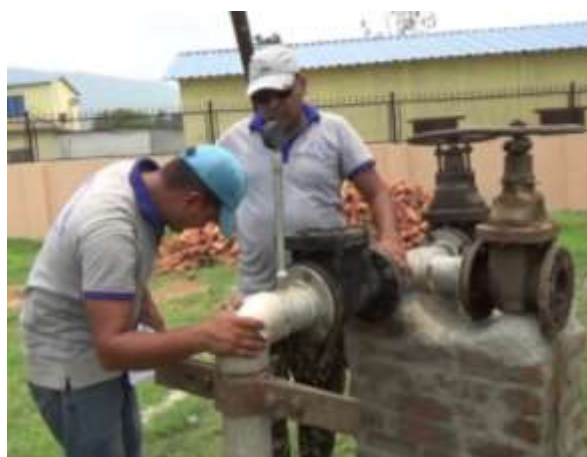
Photo 2.38 Touching Discharge Pipe
