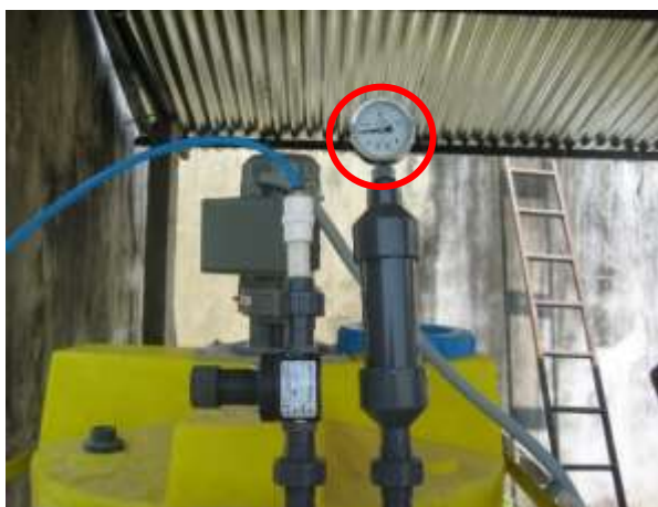
Photo 2.28 Daily Inspection of Pump (Discharge Pressure)
