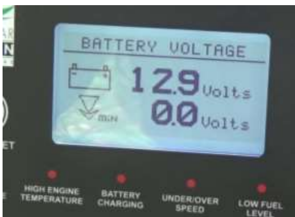
Photo 2.11 Checking Battery Condition
