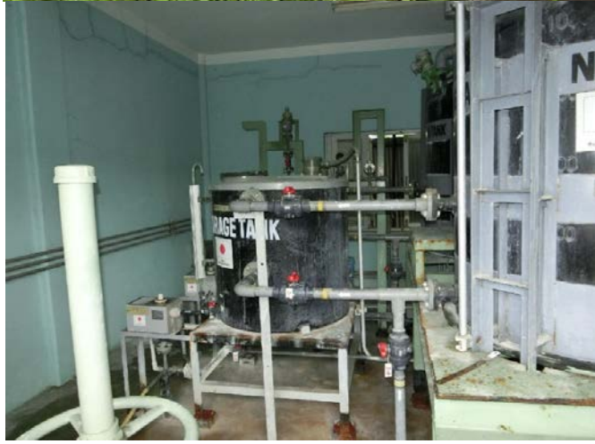
Photo-4 Mangadh WUSC on July 4 2016
