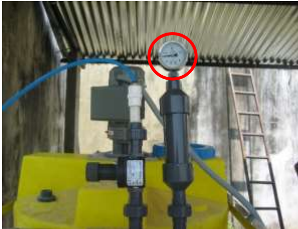
Photo-5. Daily Inspection of Pump (Discharge Pressure)
