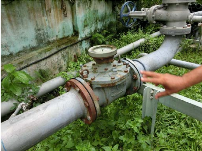
Photo-2 Mangadh WUSC on July 4 2016
