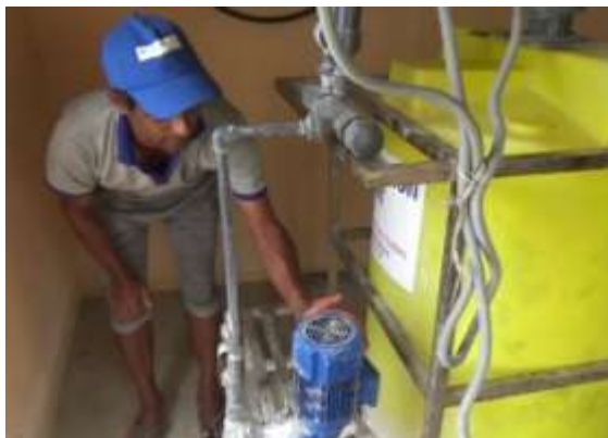
Photo-3. Daily Inspection of Pump (Heat generation)
