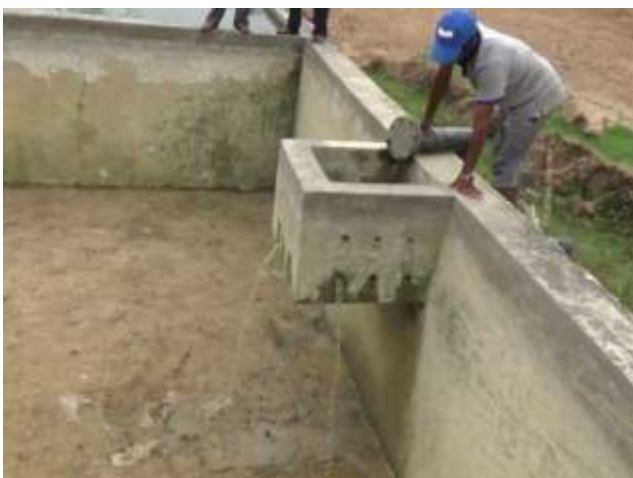
Photo-4. Filling Water to Slow Sand Filter
