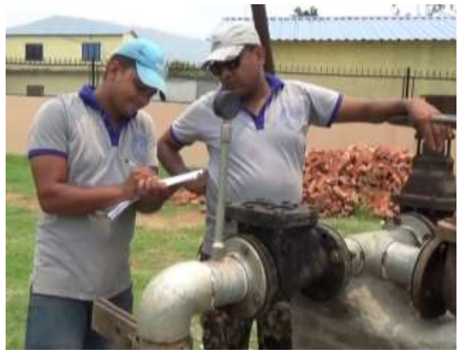
Photo-2. Checking Pressure Gauge
