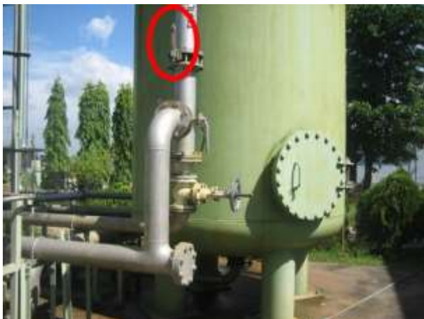
Photo 2.54 Inlet Flow Meter
