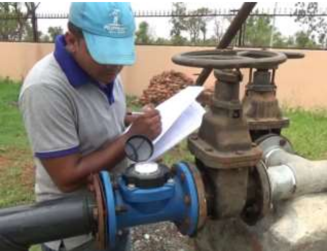
Photo-3. Checking Flow Meter
