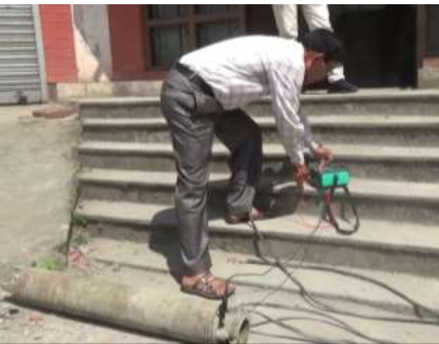
Photo-5. Measuring the Insulation Resistance Value
