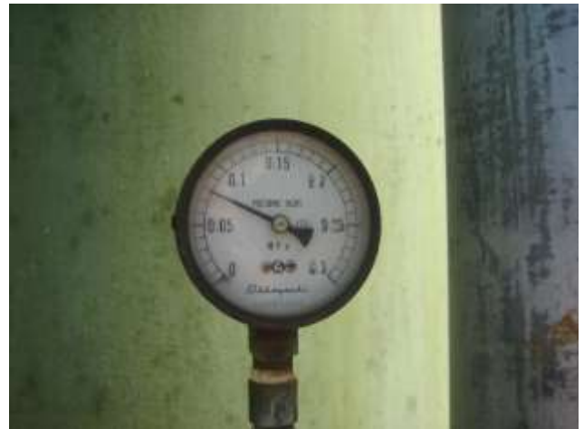
Photo-4. Pressure Gauge of Tank
