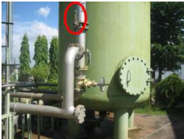
Photo 2.48 Inlet Flow Meter
