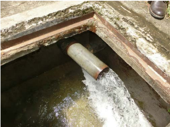
Photo-3 Besisahar WUSC on July 13, 2016 Receiving Pit inside & 2 Raw water Transmission Pipes There are NO Flow meters
