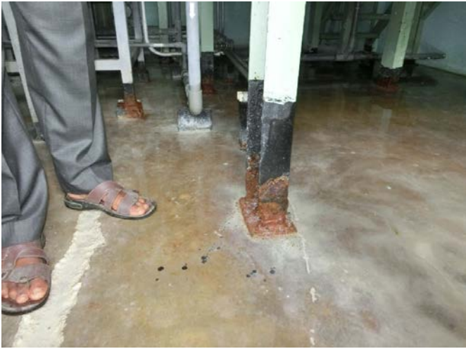
Photo-5 Mangadh WUSC on July 4 2016
