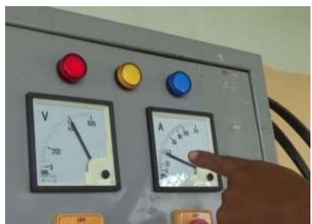
Photo 2.47 Checking Voltage and Ampere
