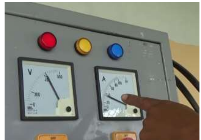
Photo-4. Checking Voltage and Ampere
