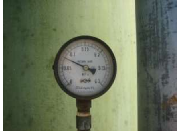
Photo 2.51 Pressure Gauge of Tank
