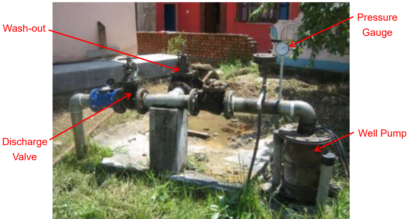
Photo-1. Typical System of the Well Pump
