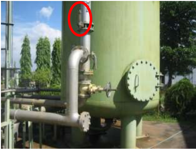
Photo-1. Inlet Flow Meter
