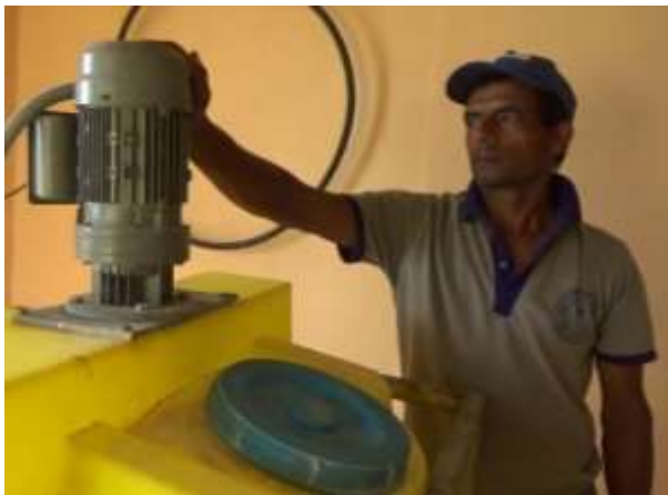
Photo 2.24 Daily Inspection of Mixer
