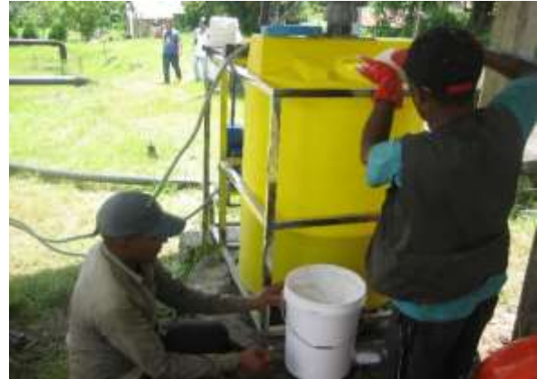
Photo 2.31 Preparation of Chlorine Solution
