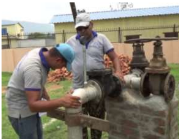
Photo 2.3. Touching Discharge Pipe
