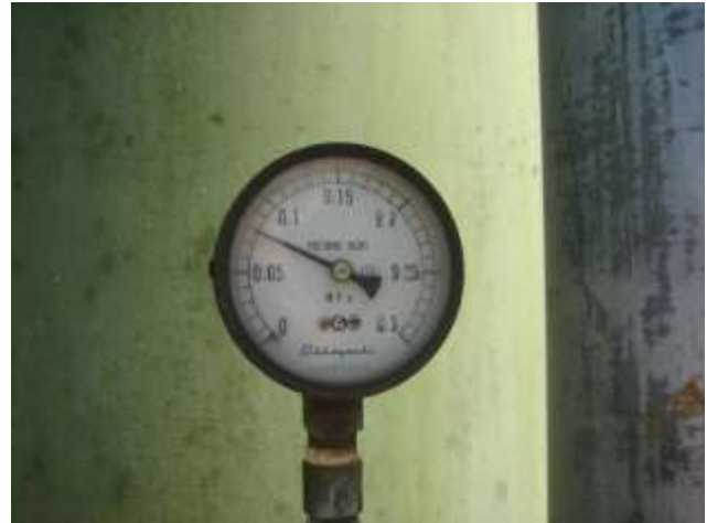
Photo-3. Pressure Gauge of Tank
