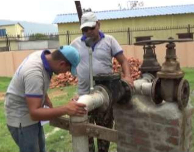
Photo-1. Touching Discharge Pipe
