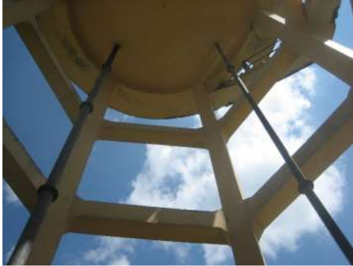
Photo 3. Sampling Point of Elevated Tank
