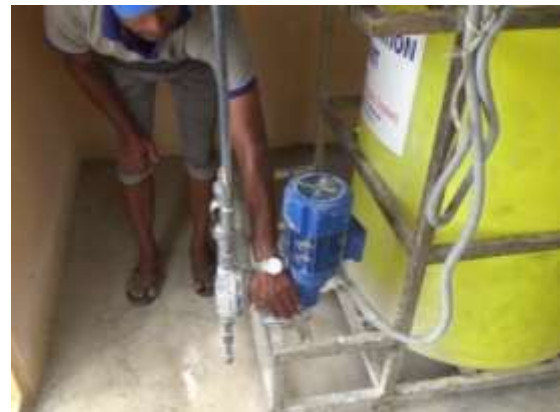
Photo-2. Daily Inspection of Pump (Abnormal noise and vibration)
