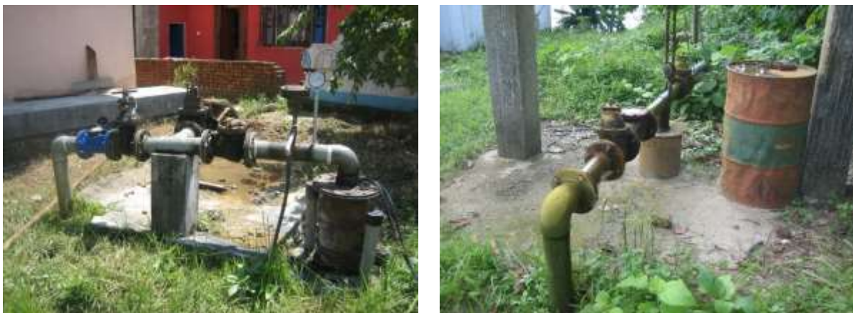
Figure 1.3 Typical Intake Structure (Left: Pragatinagar WUSC, Right: Gauradaha WUSC)
