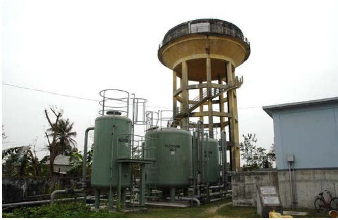
Photo-1 Mangadh WUSC on July 4 2016
