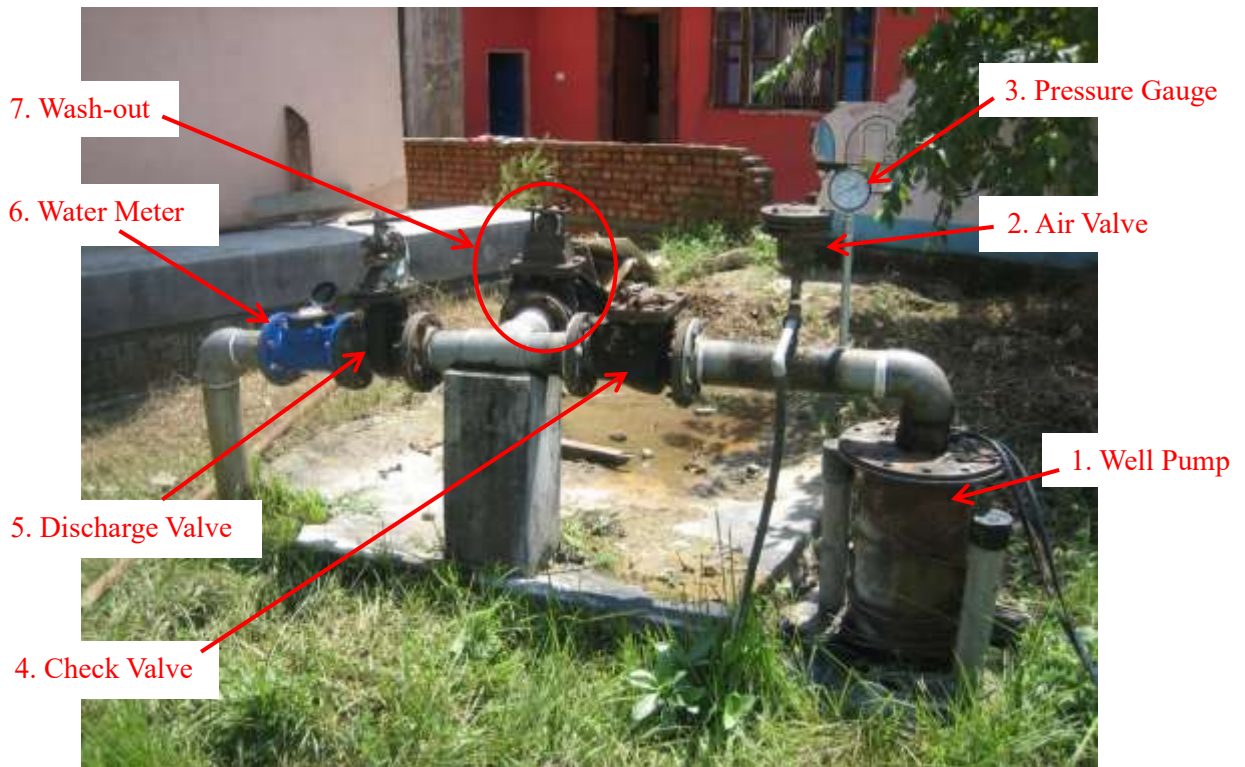
Figure 2.14 Typical System of the Well Pump
