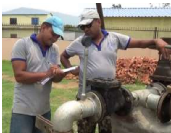
Photo 2.4. Checking Pressure Gauge
