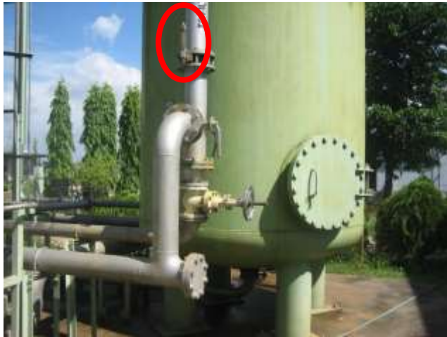
Photo-2. Inlet Flow Meter
