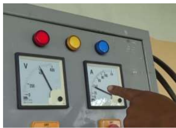
Photo 2.12 Checking Voltage and Ampere
