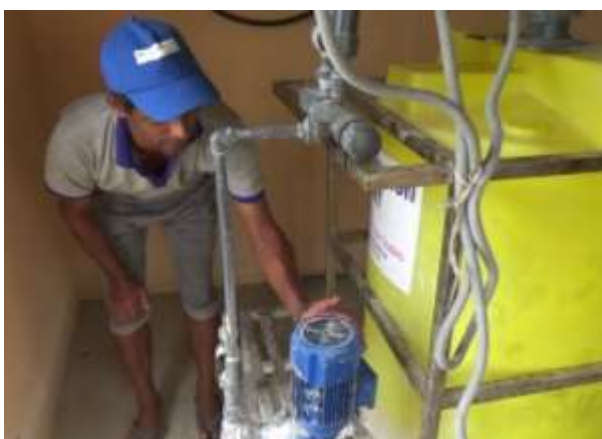
Photo 2.26 Daily Inspection of Pump (Heat generation)
