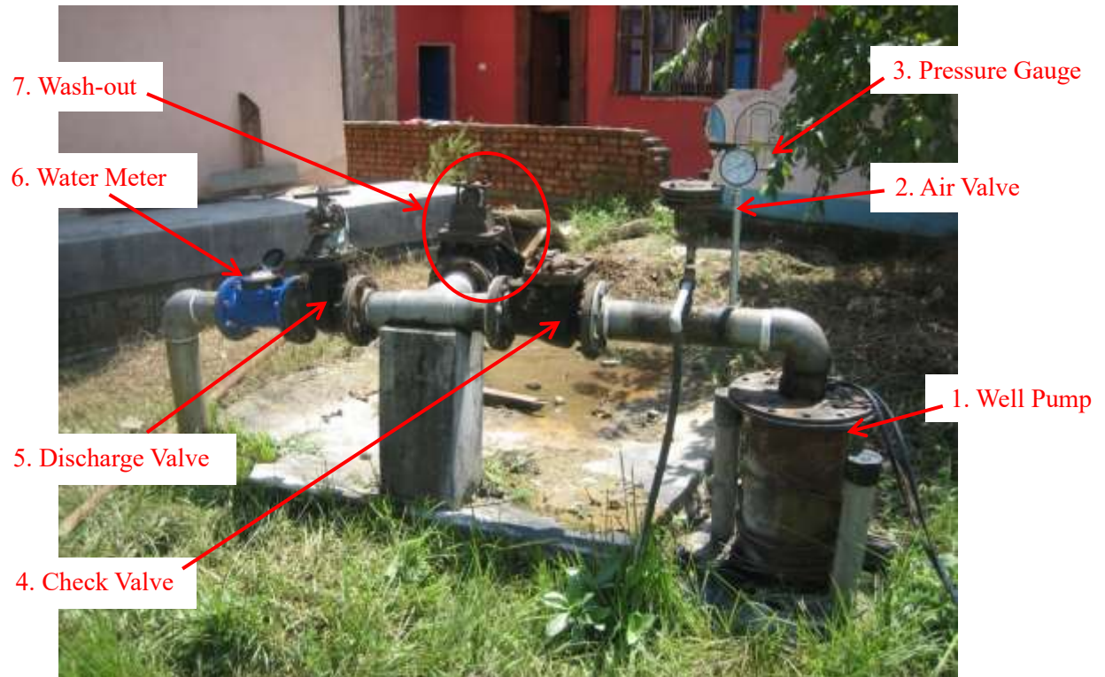
Figure 2.1 Typical System of the Well Pump
