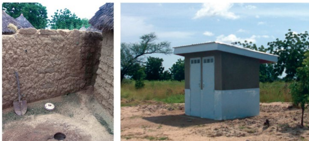
Left: Traditional latrine in the Far North Region. Right: Ventilated Improved Pit (VIP) latrines built for project to improve sanitation in the Far North Region. (Photos: Miguel Vargas-Ramirez, World Bank)
