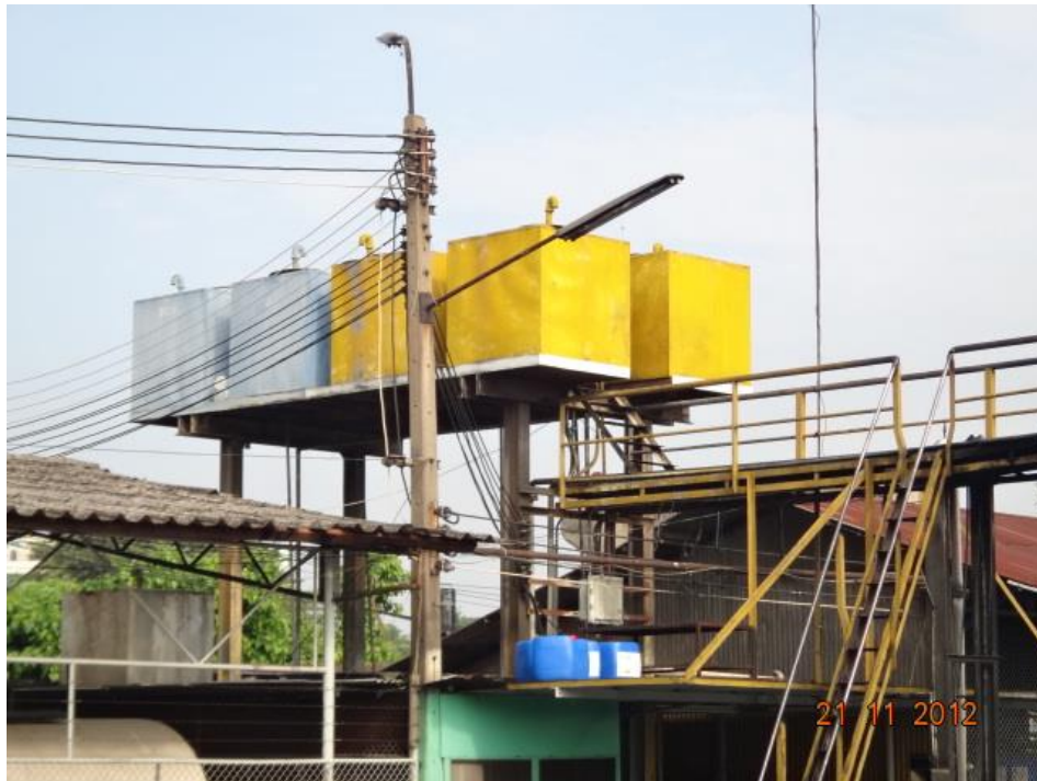
Photo. 2.4-16 Coolant Storage Tanks
