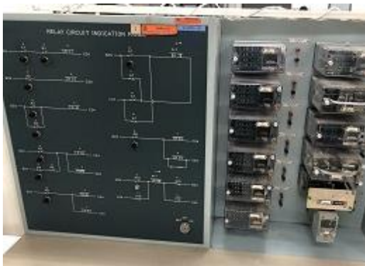
Photo. 2.4-30 Relay Interlocking Device
