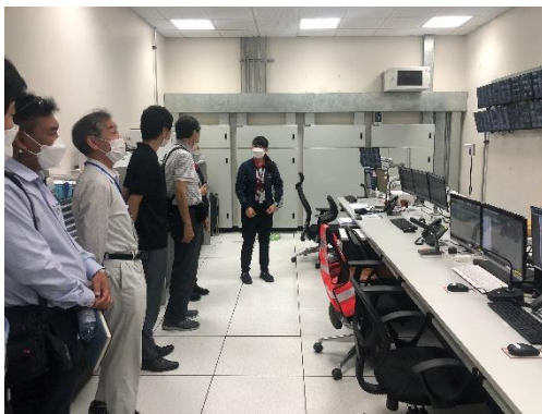
Photo. 2.4-9 Overview of Disaster Prevention room
