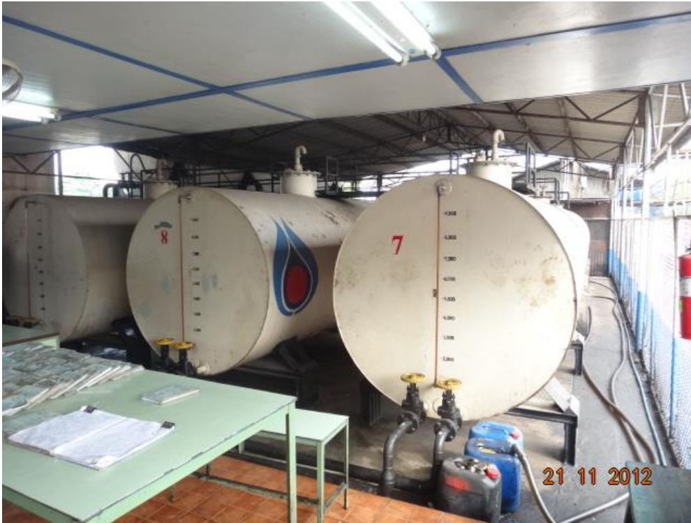
Photo. 2.4-14 Lubricant Storage Tanks
