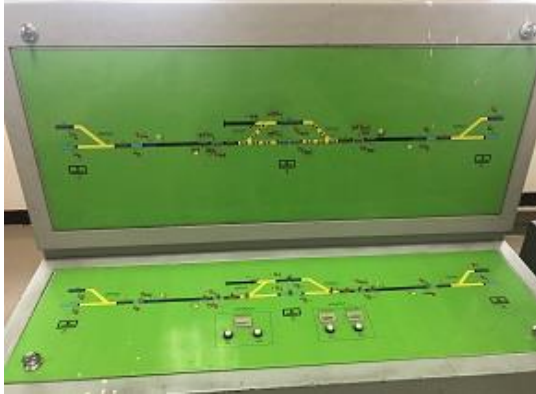
Photo. 2.4-32 Route Control Panel
