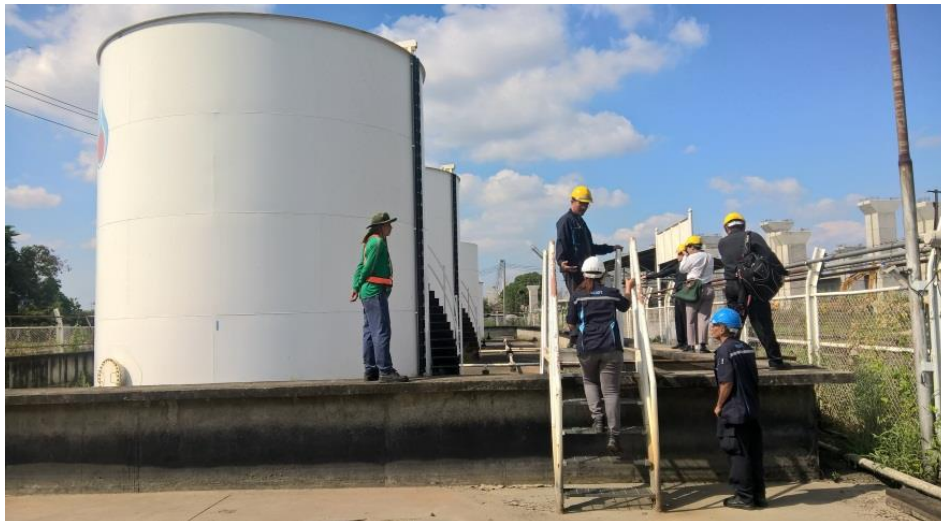
Photo. 2.4-15 Fuel Storage Tanks
