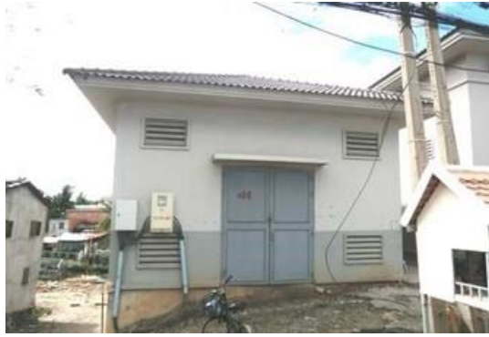
Distribution Substation D005AD005
