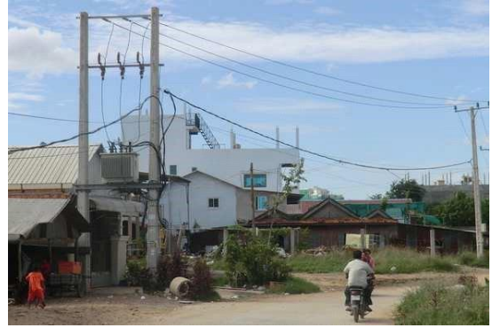
Pole Transformer P1217
