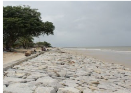
Figure 4-86 Natural Stone Revetment Pengaman Pantai Pulau Rupert Kab.Bengkalis BWS SUMATERA III RIAU, 2011
