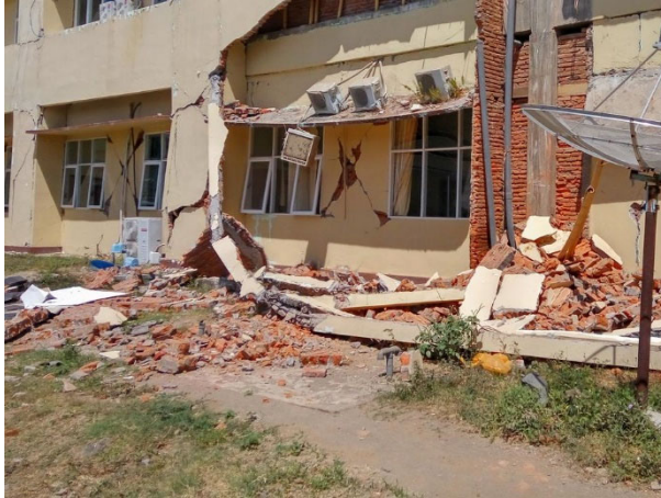
Figure 2-10 Damaged Public Hospital (RSUD) Tanjung, North Lombok District (no more function)
