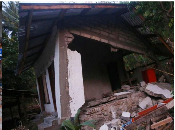
Figure 2-15 Collapsed house due to poor construction methods (2)
