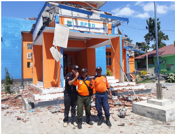
Figure 2-12 Partially damaged Office of BPBD North Lombok District
