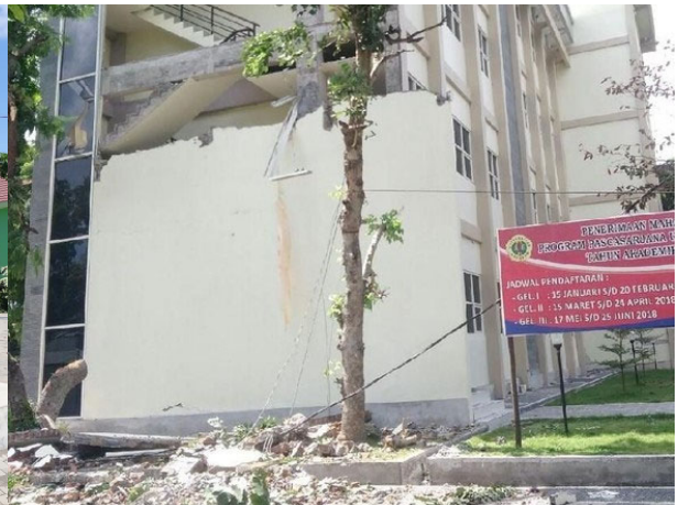
Figure 2-13 Partially damage of building in Mataram University
