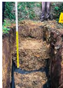
After backfilling by clay soil. Filling is only halfway for demonstration purpose. The clay soil layer has not compacted to surface level (125.5m) yet to avoid collapsing.
