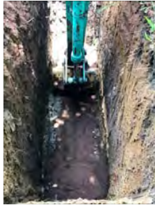
Filling the second layer on top of first PRB layer (~0.5m and compaction by excavator bucket).
