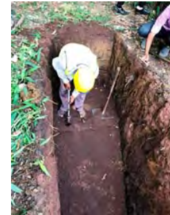
Core sampling on the finished layer (S4, S5, S6). The finished section was having a width of 1.10m and length of 1.5m.
