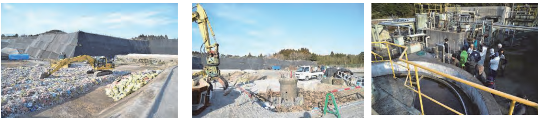
Sanitary Landfill Site and Leachate treatment facility
