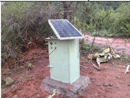
The solar panel and the power box
