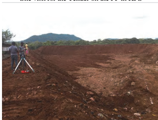
Earth works at the landfill site, after removal of hard rocks (May 2018)
