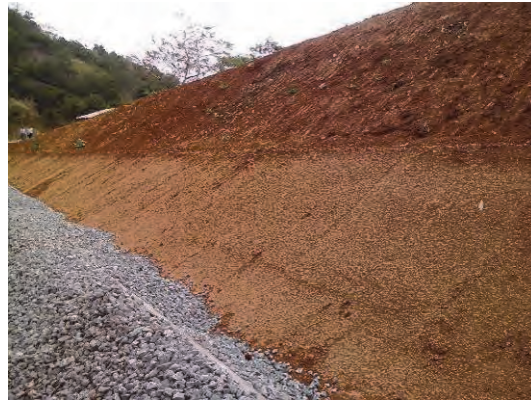
The bentonite-soil mixed liner on the inside slope of the landfill site
