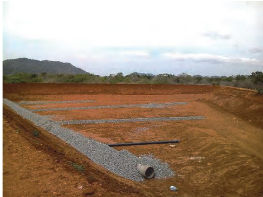
Leachate pipe networks
