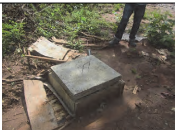
Protected monitoring well damaged by elephant
