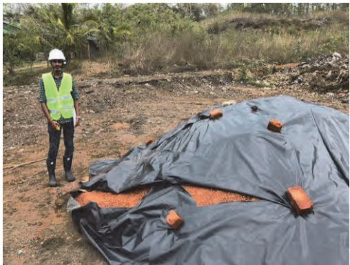
Material of PRB in the dumpsite of KMC
