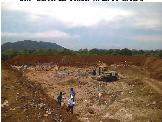
Earth works at the landfill site, before removal of hard rocks (May 2018)
