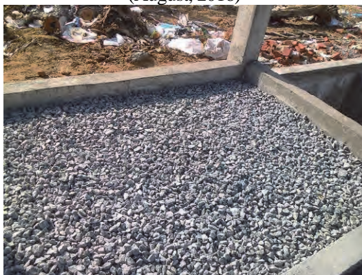
Sludge drying bed (August, 2018)
