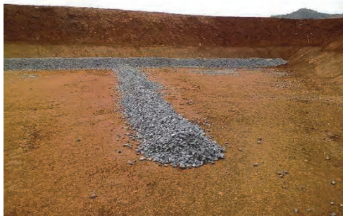
Branch line pipe (covered by aggregates)
