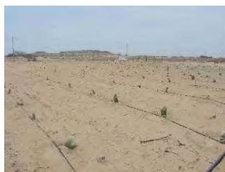
Removal of P. juliflora in the target area and installation of drip irrigation
