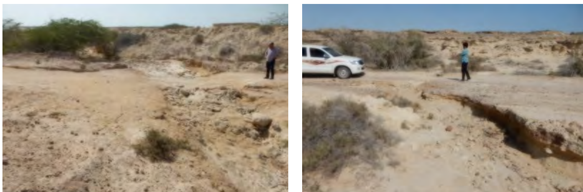
5035 Damaged by Erosion
