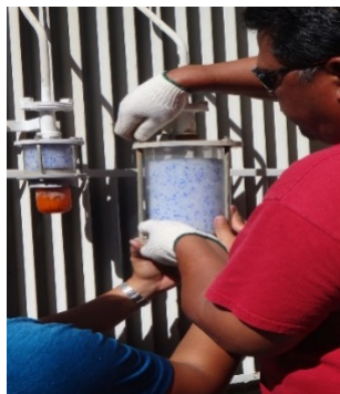
Figure 9-2-8.3 Silica gel replacement
