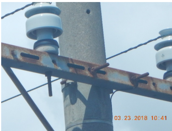
(a) Rusting arm brace
