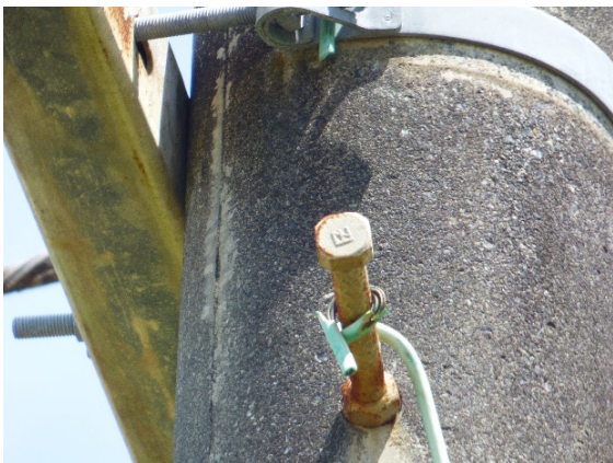
Figure 9-1-5-1.6 Disconnected grounding wire
