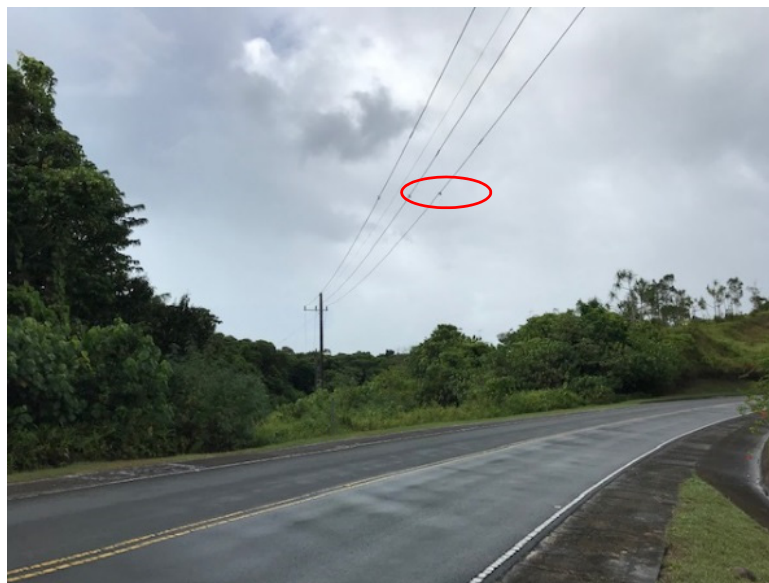
Figure 9-1-4-1.11 Example of overcurrent indicators installed (line around Kokusai substation)
