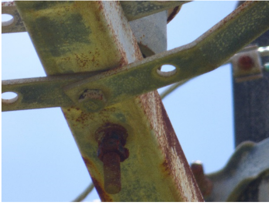
Figure 9-1-5-1.2 Loosening of the nut for the insulator
