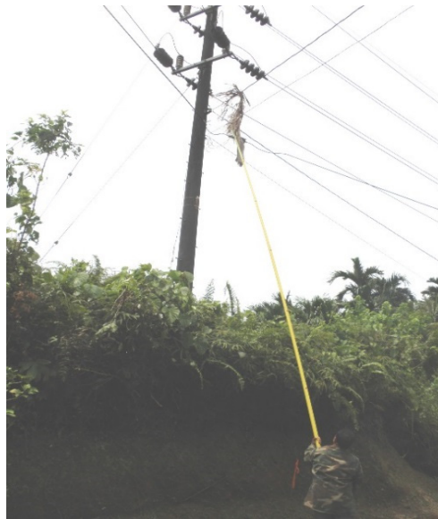
Figure 9-1-4-1.12 Windblown branch (cause of a fault)
