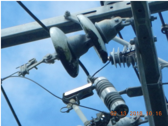
Figure 9-1-5-1.4 Equipment damage (arrester)
