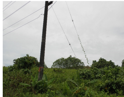
Figure 9-1-4-1.8 Growth on guy wires without a vine guard
