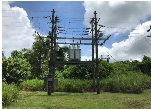
Figure 6-1-1-2.2 Example of pole-mounted substation equipment (Asahi Substation)
