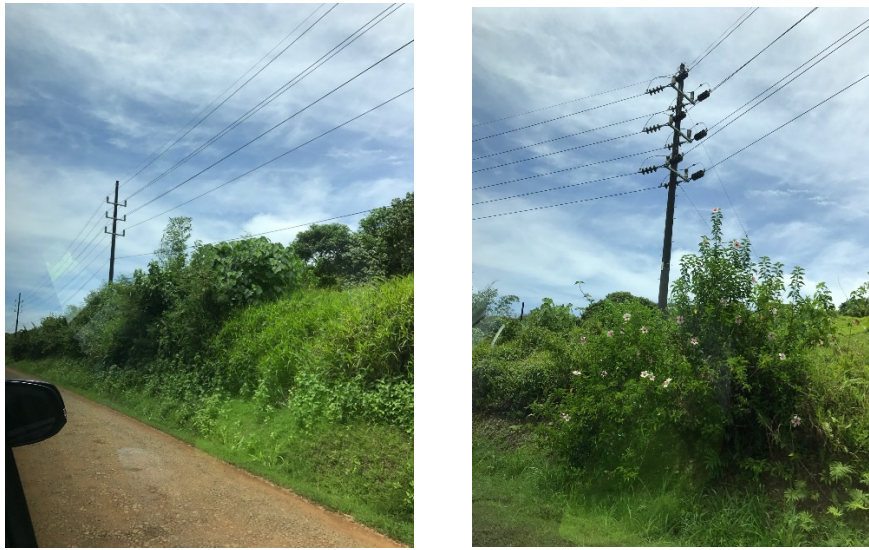
Figure. 6-1-1-5.2 Status of transmission line mounting on poles in the double-circuit section (Between Aimeliik power station and Nekken substation)
