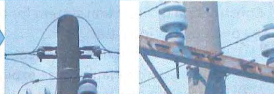
Corrosion rupture of clevis
