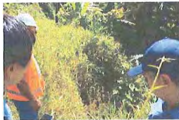
The old road where land slipped
