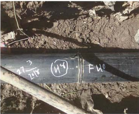
Joint # 48 Location IP3 +837' Straight Date 27-Mar
