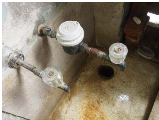
Situation of Groundwater Dependent Type (In-home piping connect to groundwater pump)
