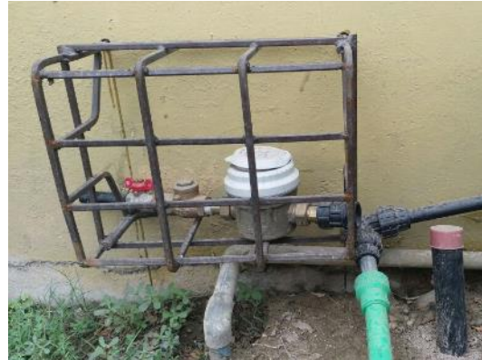
Bypassing due to meter stuck
