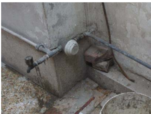
Meter installation in landscape direction
