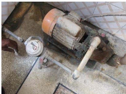
Situation of Illegal Pump Suction
