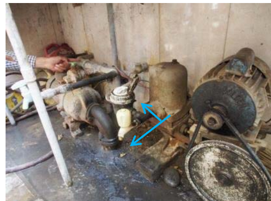
Meter installation after the branch
