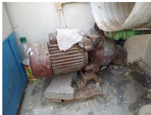
Groundwater Pump (It is provided by electric company cheaply)
