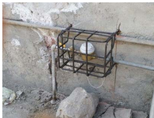
Meter installation (on the wall)
