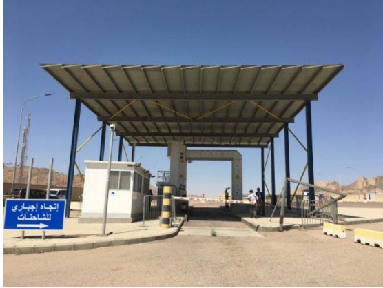
Portal type X-ray inspection machine deployed at Yard-4
