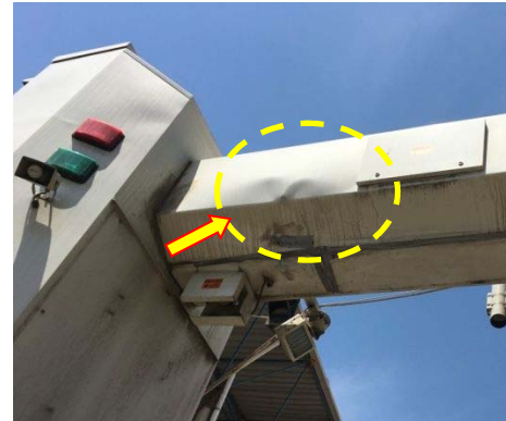
Damaged part (contacted by a cargo during X-ray inspection)
