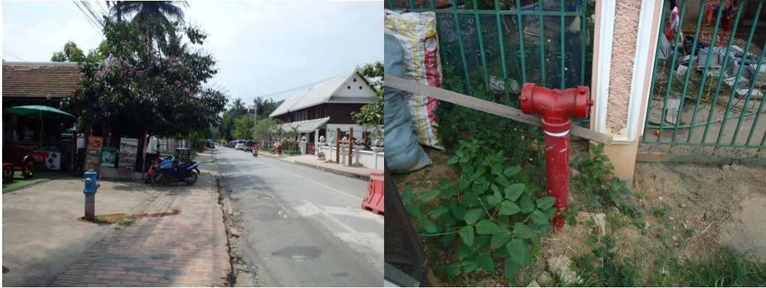
Photo 2.2.4 Fire hydrants installed in the World Heritage Site and in the city area (Left; World Heritage Site, Right; city area)
