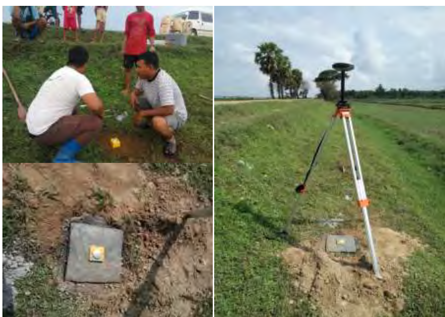
Figure 8 the BM installed at the feasibility study. Source: AAS MM
