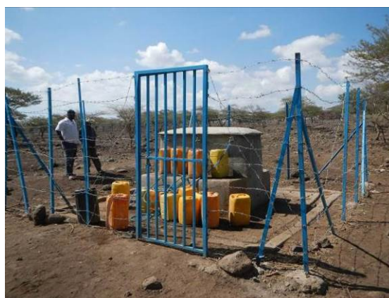
Figure 1-52 Public fountains constructed by other donors
