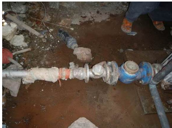
Figure 1-43 Pipeline around the pump
