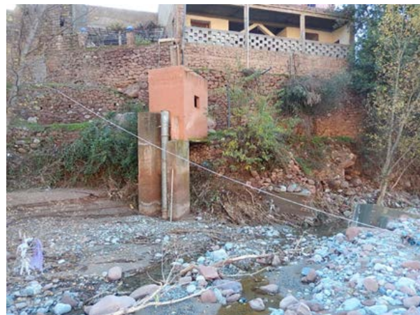
Photo 2.3.2 Abandoned Water Level Gauge
