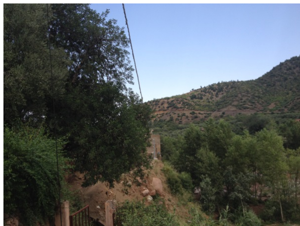
10 th July Installation of cable and wire (between 3m pole and 5m pole)
