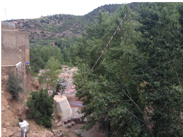
10 th July Installation of cable and wire (between arm and 3m pole)
