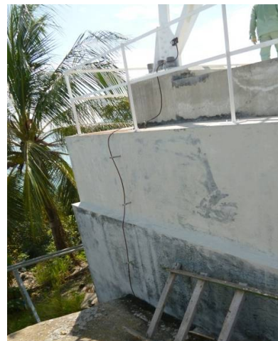
(2) Earth Terminal at Steel Tower Leg
