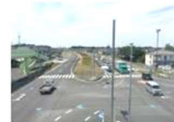
Construction from outside of ROW with service road as the border of ROW
