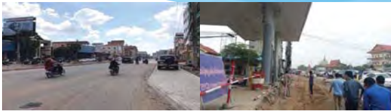
House not properly demolish if without the inspection of the MPWT
