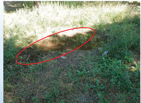
Leakage from Distribution Pipes
