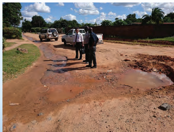
Leakage from Distribution Pipes
