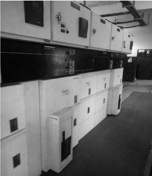
Existing Transformer 2*7.5MVA 33/11kv
