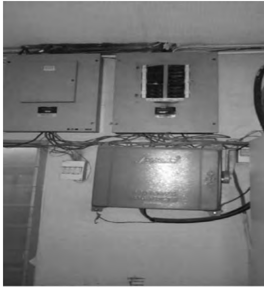
Existing 100AMP Change Over Panel
