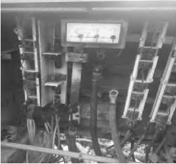
Existing Feeder pillar
