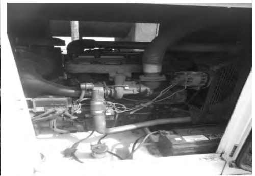
Existing Generator 1Unit1*500KVA
