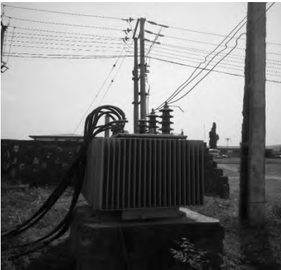
Existing Transformer 2*500KVA, 33/0.415KV
