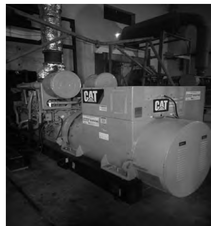
Existing Generator 1Unit, total output is 6MW
