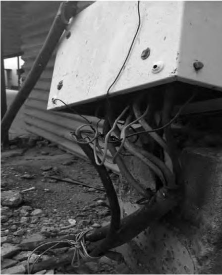
Existing connector switch 7.5MVA 33/11kv
