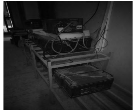
Existing inverter battery
