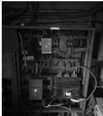
Existing Feeder pillar
