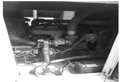
Existing Generator 1Unit 1*500KVA
