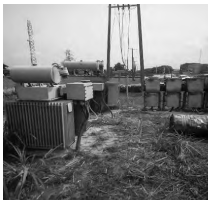
Existing Transformer 2*500KVA 11/0.415KV
