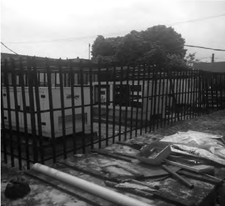
Existing Generator 3Units, 2Units (1*27KVA, 415V、1*20KVA, 415V) Available
