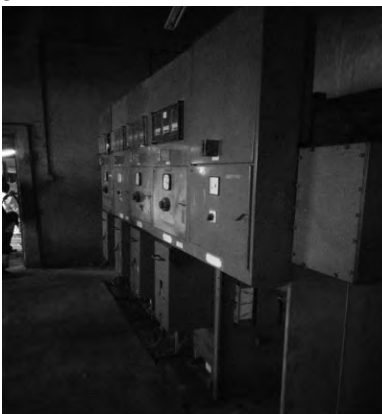
Existing Transformer 7.5MVA 33/11kv
