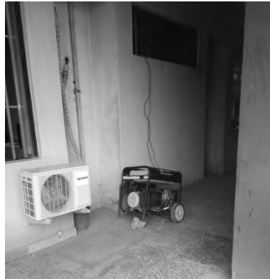
Existing Generator for the laboratory 1*2.5KVA, 220/240V
