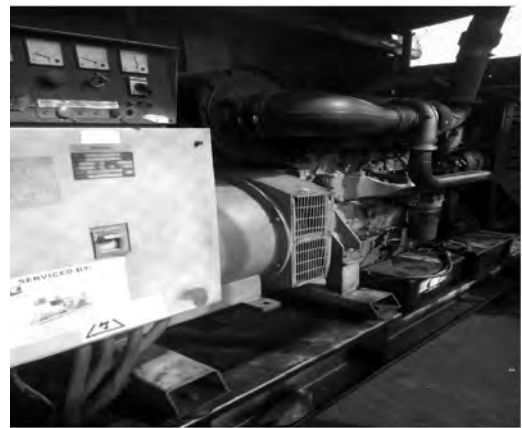
Existing Generator 1Unit 1*500KVA
