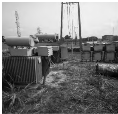
Existing Transformer 2*500KVA 11/0.415KV
