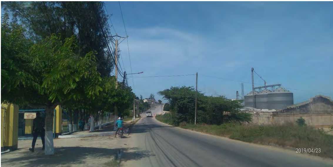
Low voltage power distribution line 6 (At the paved road to the site)
