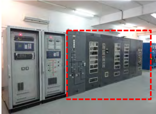
Photograph 2-8 Old Control Panels (Planned Space for Installing the New Protection/Control Panel)
