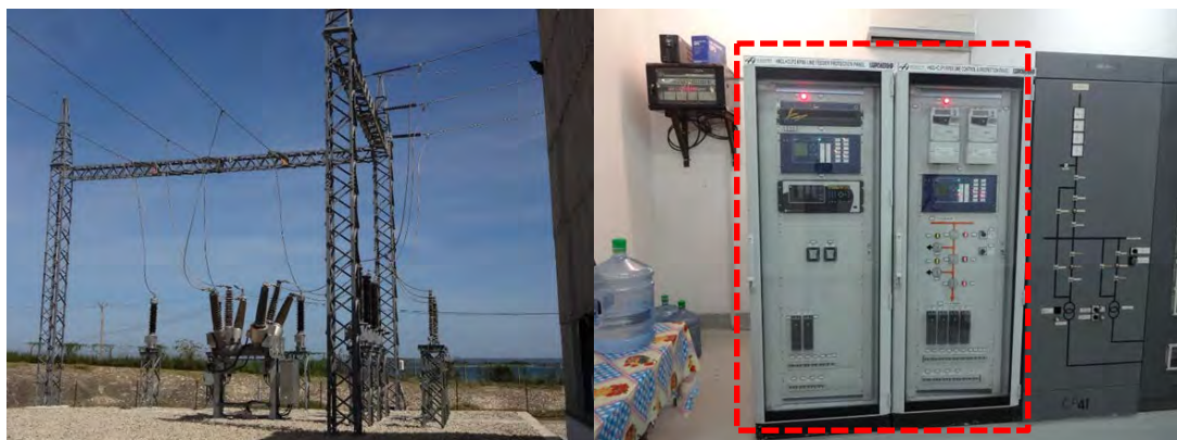
Photograph 2-2 Power Receiving Switchgear for the Barge, and Protection and Control Panels
