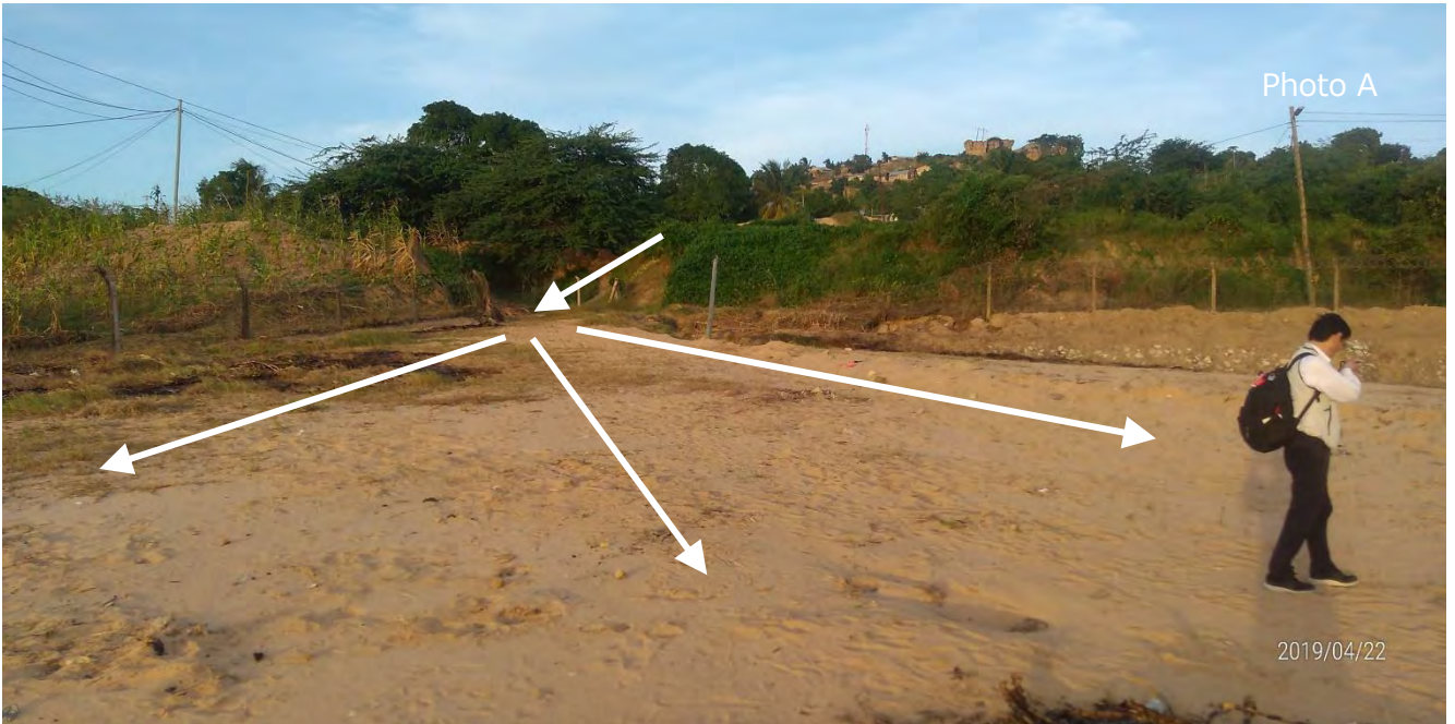
Plenty of soil was flown into the free space at east side of the old generator building. Its thickness almost reaches human height.
