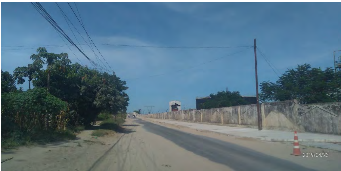
Low voltage power distribution line 7 (At the paved road to the site)
