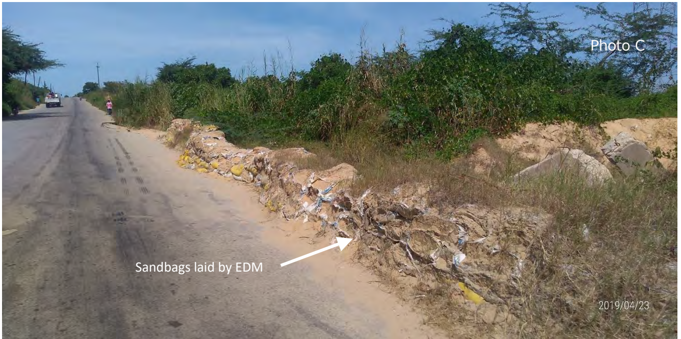
EDM laid sandbags as an emergency measure, however, they are now damaged most probably by UV light and it needs to be restored.
