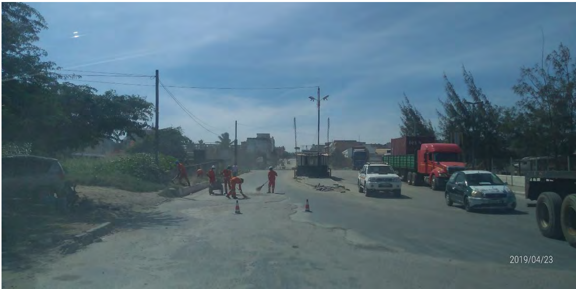
Low voltage power distribution line 3 (In front of the Roundabout)
