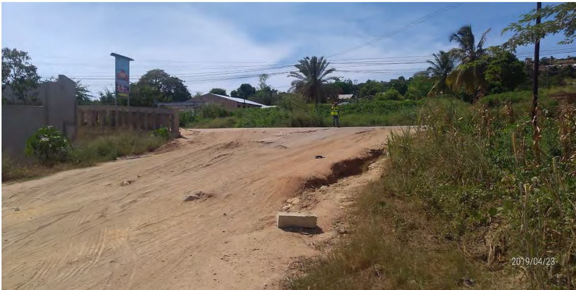
Unpaved road at north side of the site 1 (surface is uneven and rough)
