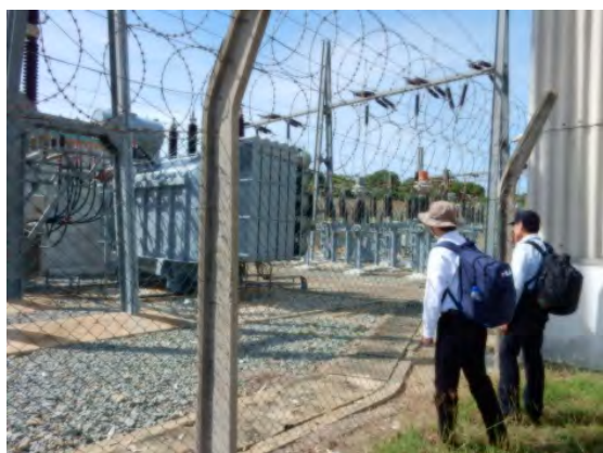
Photograph-5 Existing switchgear in Nacala substation
