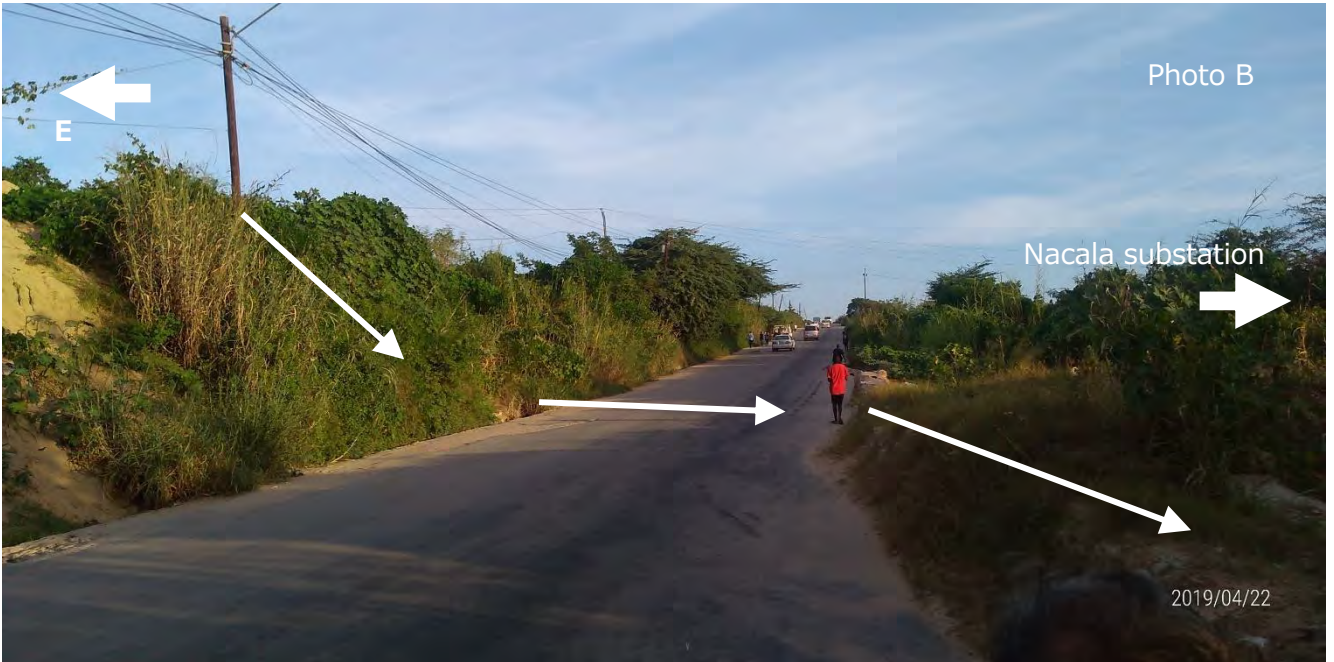
Road at east side of the substation of which level is higher than the substation. Fine sandy soil eroded and flown out from the higher land at east side of this road flown into the substation.
