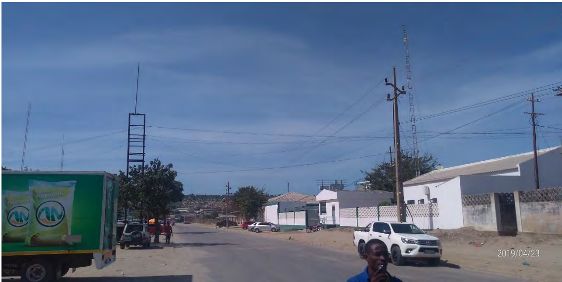
Low voltage power distribution line 1 (between Nacala Port and the Roundabout)
