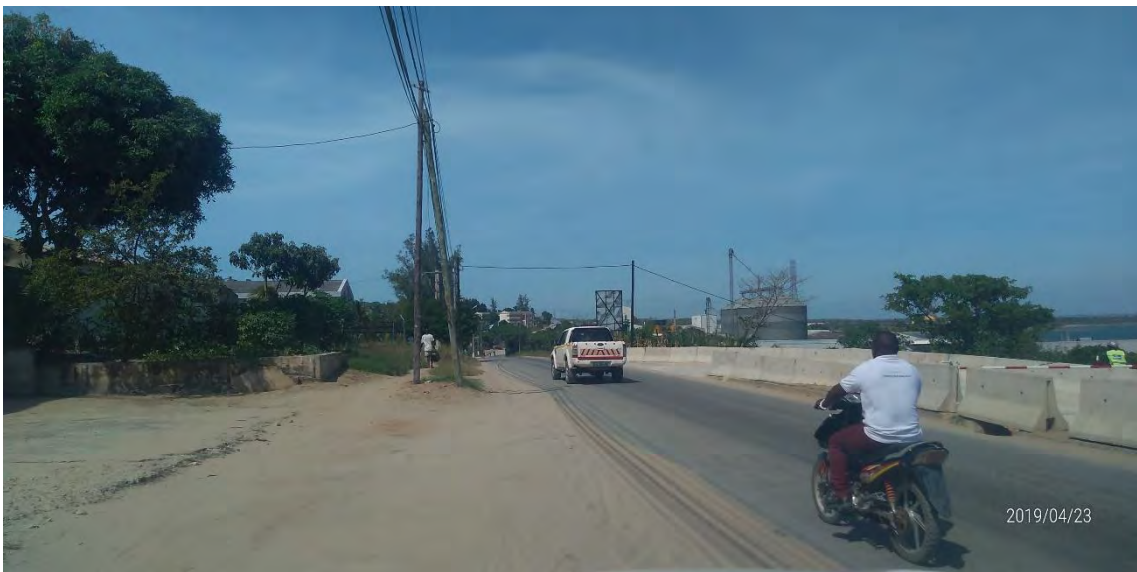
Low voltage power distribution line 5 (At the paved road to the site)
