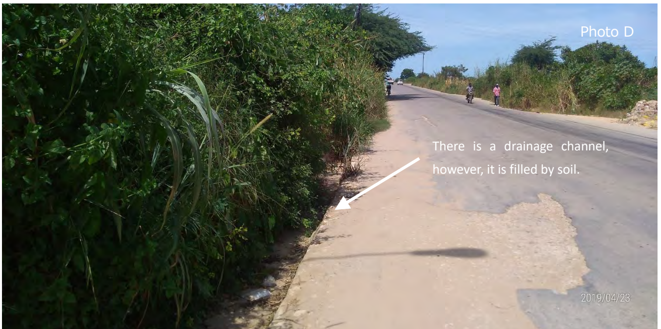
There is a drainage channel at east side of the road, however, it is filled by soil and seems not functioning.
