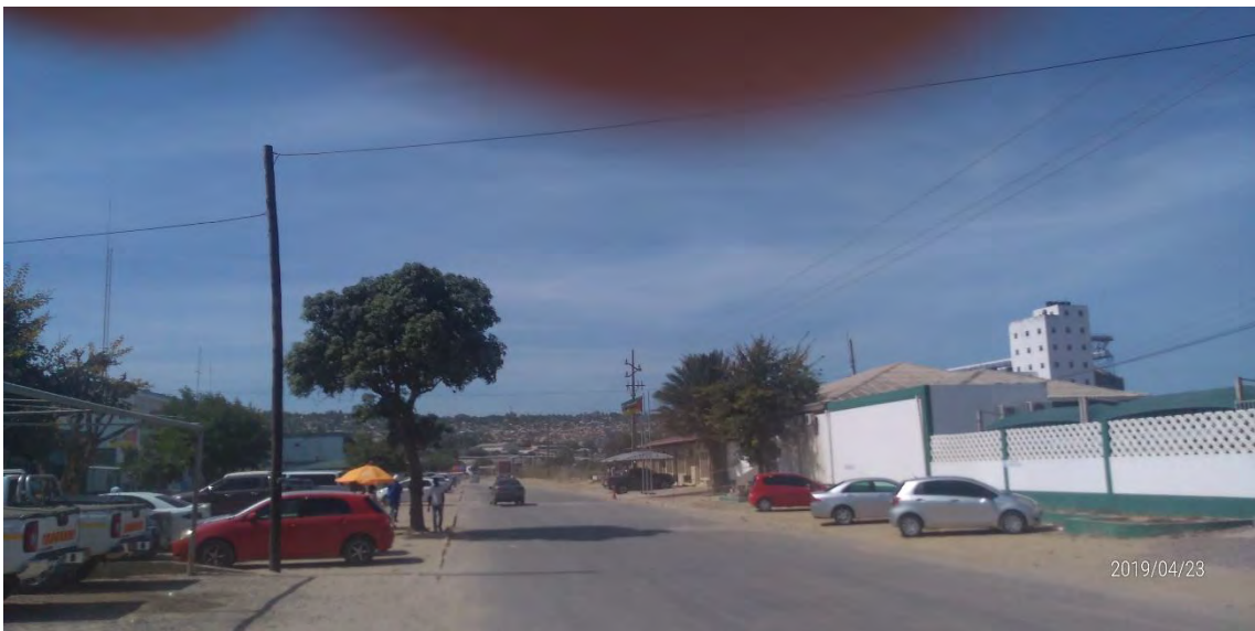
Low voltage power distribution line 2 (between Nacala Port and the Roundabout)
