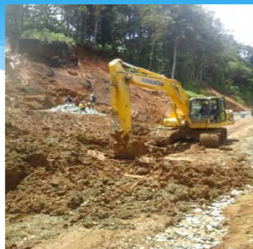
Due to landslip at Ch. 1+000 , constructing of gabion basket for the slip protection at Mt. Kuta.
