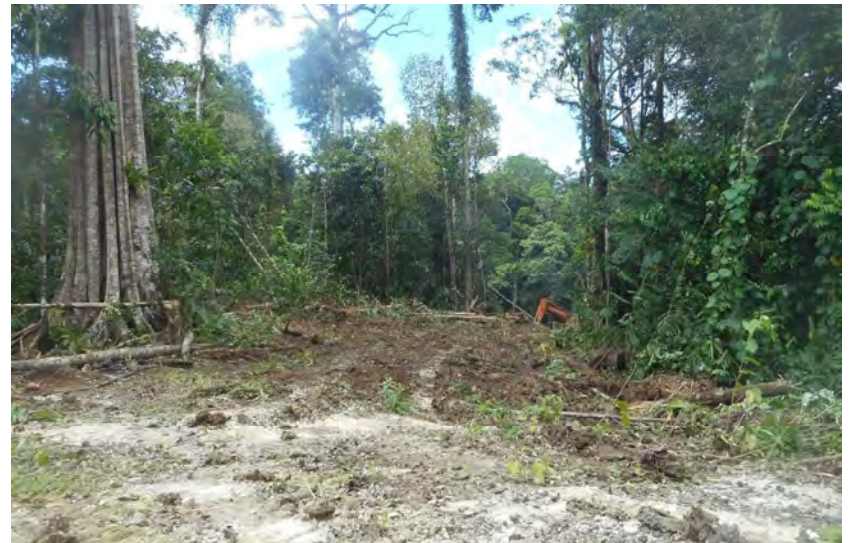
End of existing logging road at Vol River – Kandrian approach (photo after) Road connected...!!!
