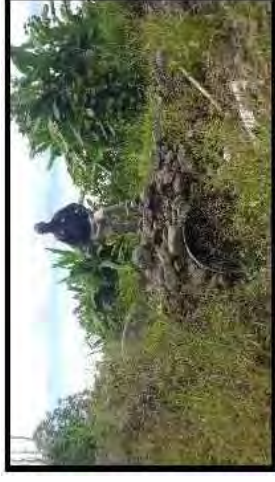
Fig 1: @ Ch: 15 – 500 (750mm X 10m dia. CSP cross culvert laid last year, July (2016). No head wall constructed. Over growth of vegetation around the inlet and outlet. Will cause overflow if heavy flooding occurs.
