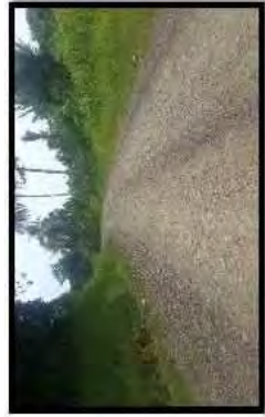
Fig. 3: Ck: 22+ 200 showing condition of a section of the road before and after.
