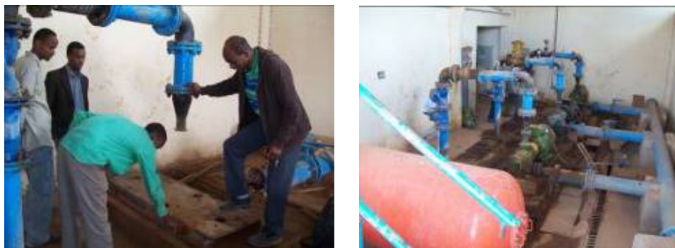
Figure 2.4: Installation of the surface pump (left) and General View of Conveyance Pump Station
