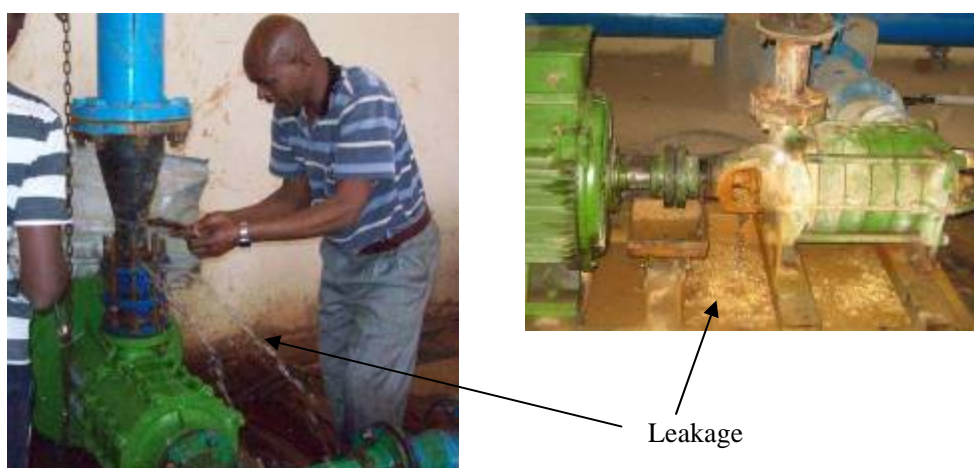
Leakage at the time of replacement (left) and during regular operation (right)
