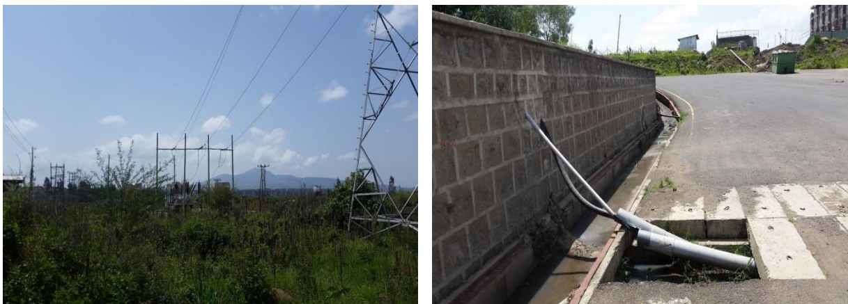
Picture 3: Existing Mobile Sub-Station and Improper Cable Installation
