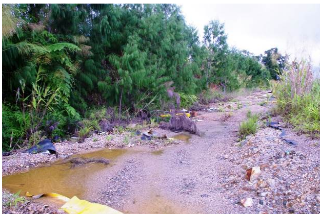
Photo. 3 Seepage beside of Heap
