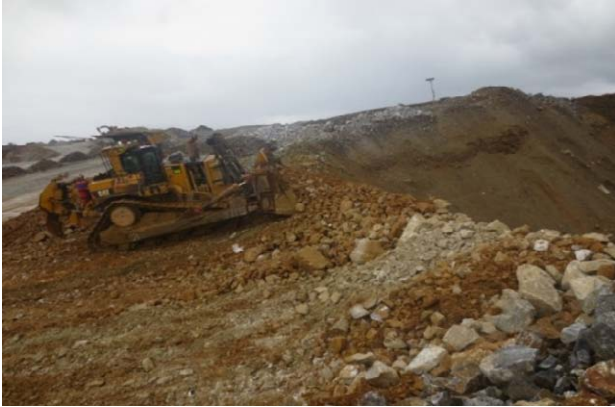
Photo 3: Dozer pushing waste rocks over natural cliff at Ok Tedi Mine, Western Province
