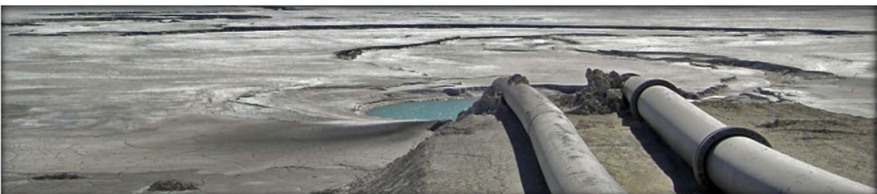
Photo 6: Tailings Pipeline Facilities
