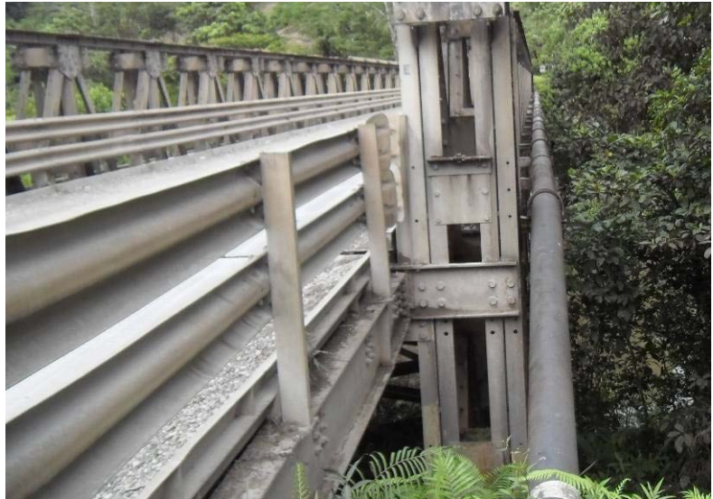
Copper concentrate pipeline (left) and a larger pyrite concentrate pipeline (right) at the Ok Menga bridge
