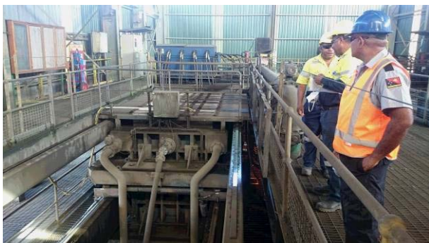
Filter press at the Kiunga operation center
