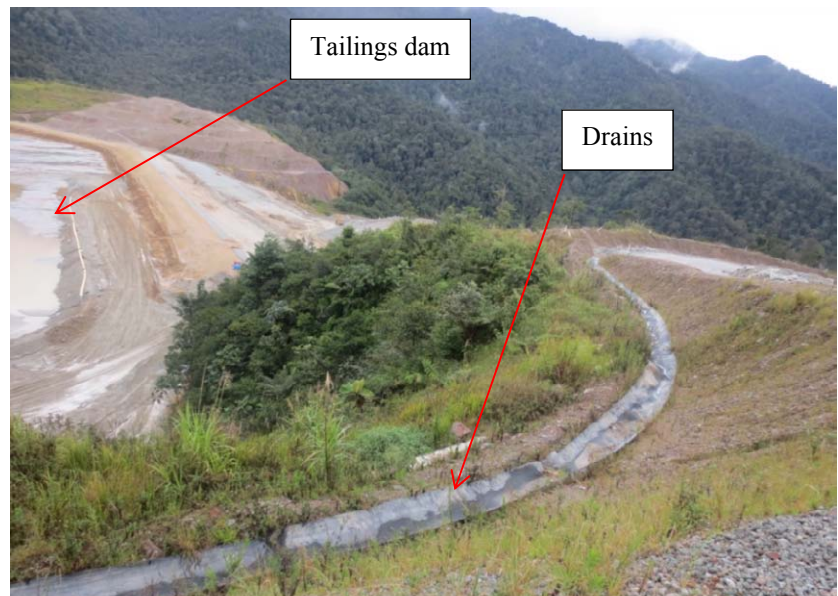
Photo 4: Diversion drain channeling access water into the Tailings dam at Hidden Valley Mine, Morobe Province
